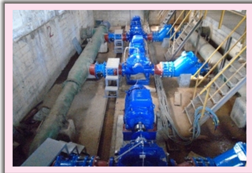
PUMPS, PANELS AND ACCESSORIES INSTALLED AT SULEJA WATER WORKS
