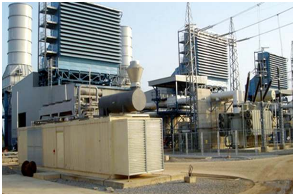
Figure 35: Power Distribution in Nigeria
