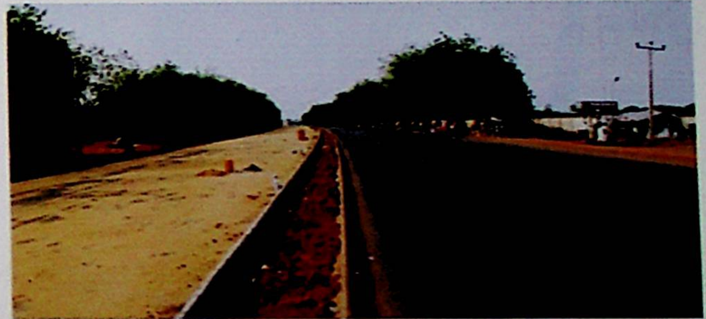
On-going multi billion naira tripartition of Gidan Man-ada to Airport road by Gov Wamakko
