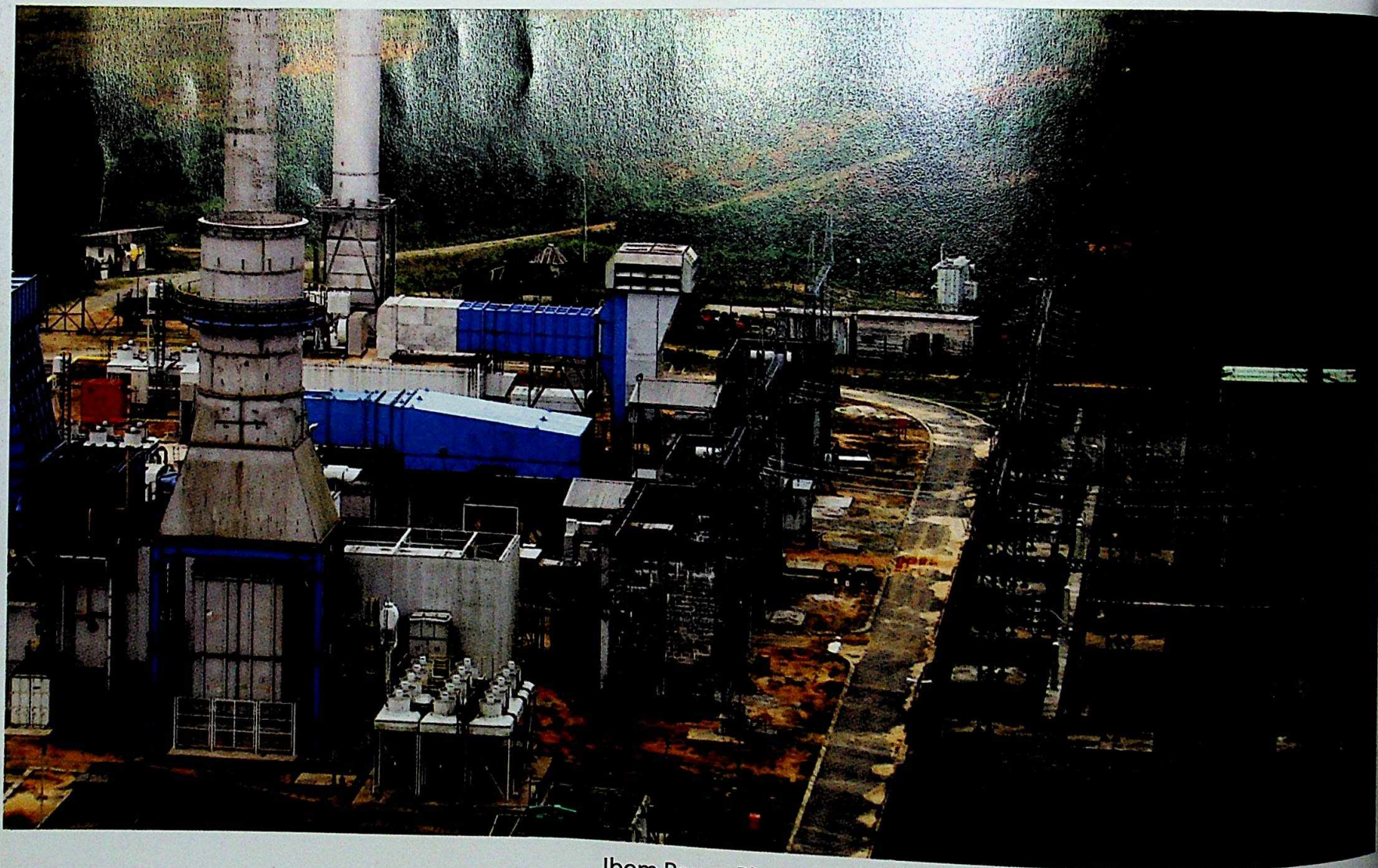
Ibom Power Plant
