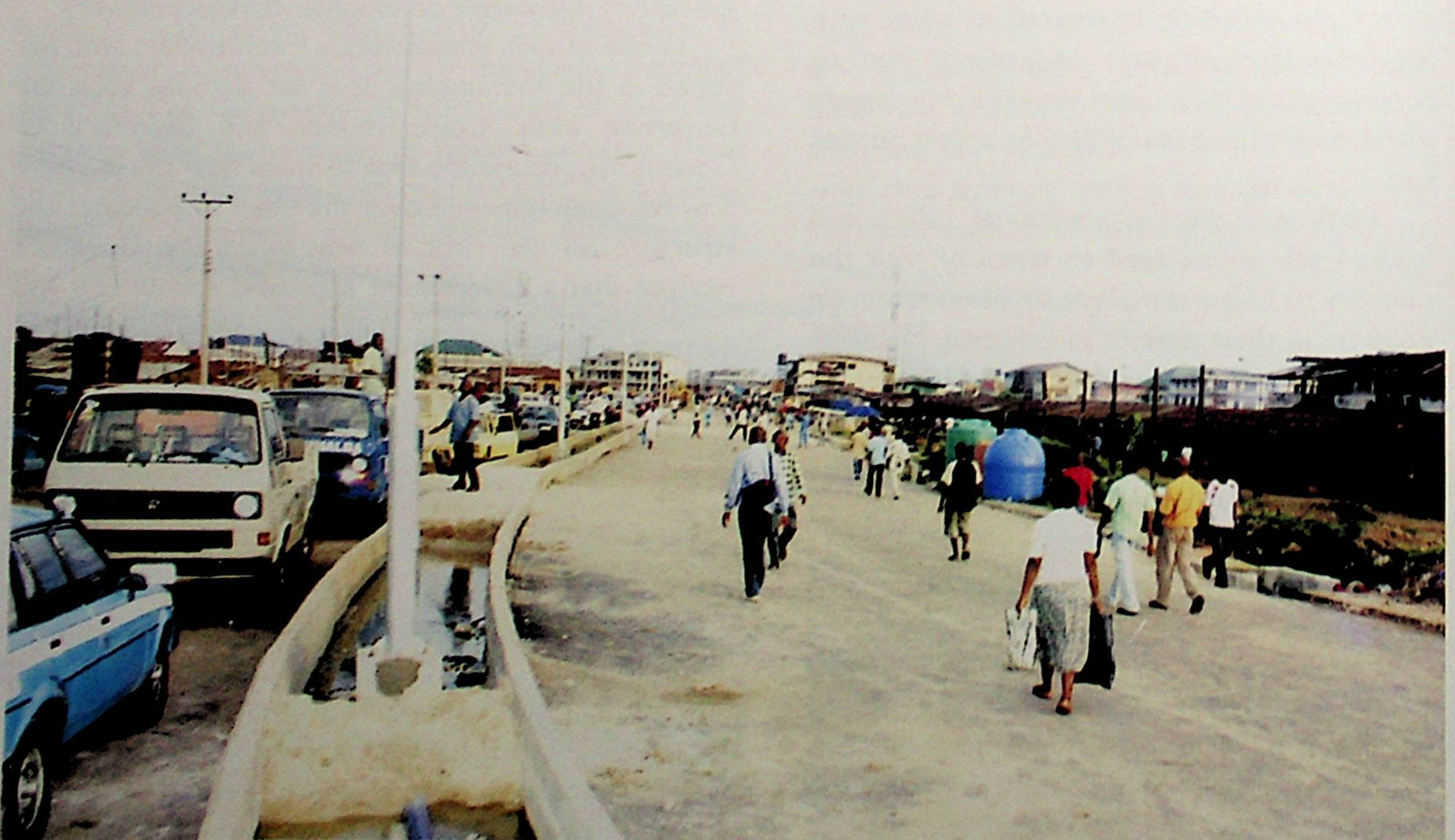
Work in progress on the Abuja by pass mile 3 road, Port Harcourt
