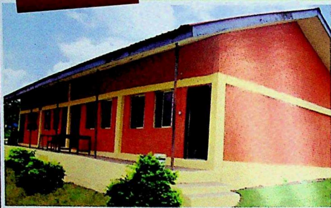
The Newly Renovated Administrative Block (A) Salvaged from total Collapse, at Co-operative College, Ijeja - Abeokuta
