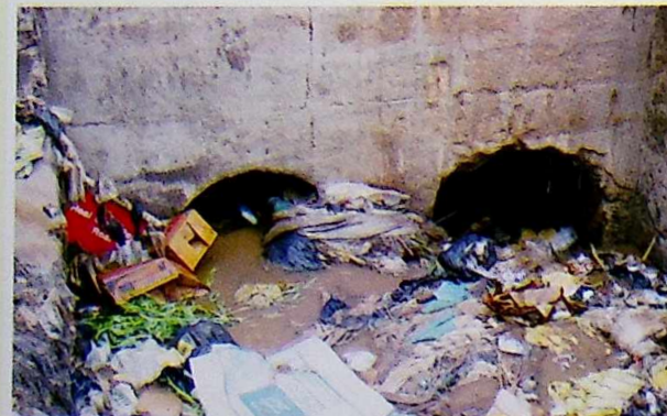
A Blocked Water Way At Gbangba Area, Abeokuta
