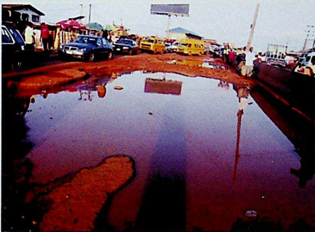
Lagos-Abeokuta Expressway Road (Before Rehabilitation)
