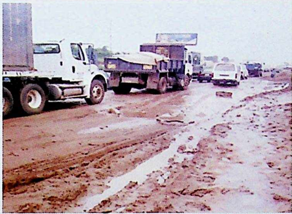
Lagos-Ibadan Expressway (before rehabilitation)
