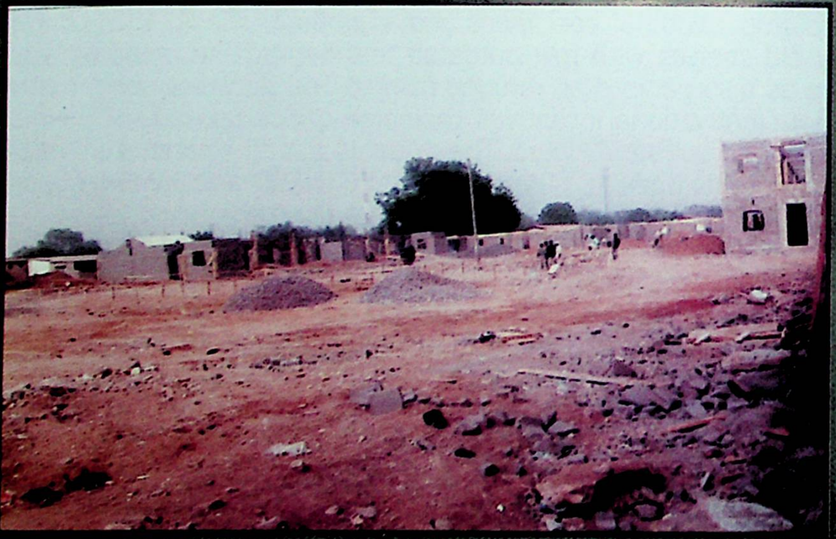
Famous Sa'ad Zungur Primary School Bauchi Phase I&II undergoing construction, while Phase III is in a foundation stage.
