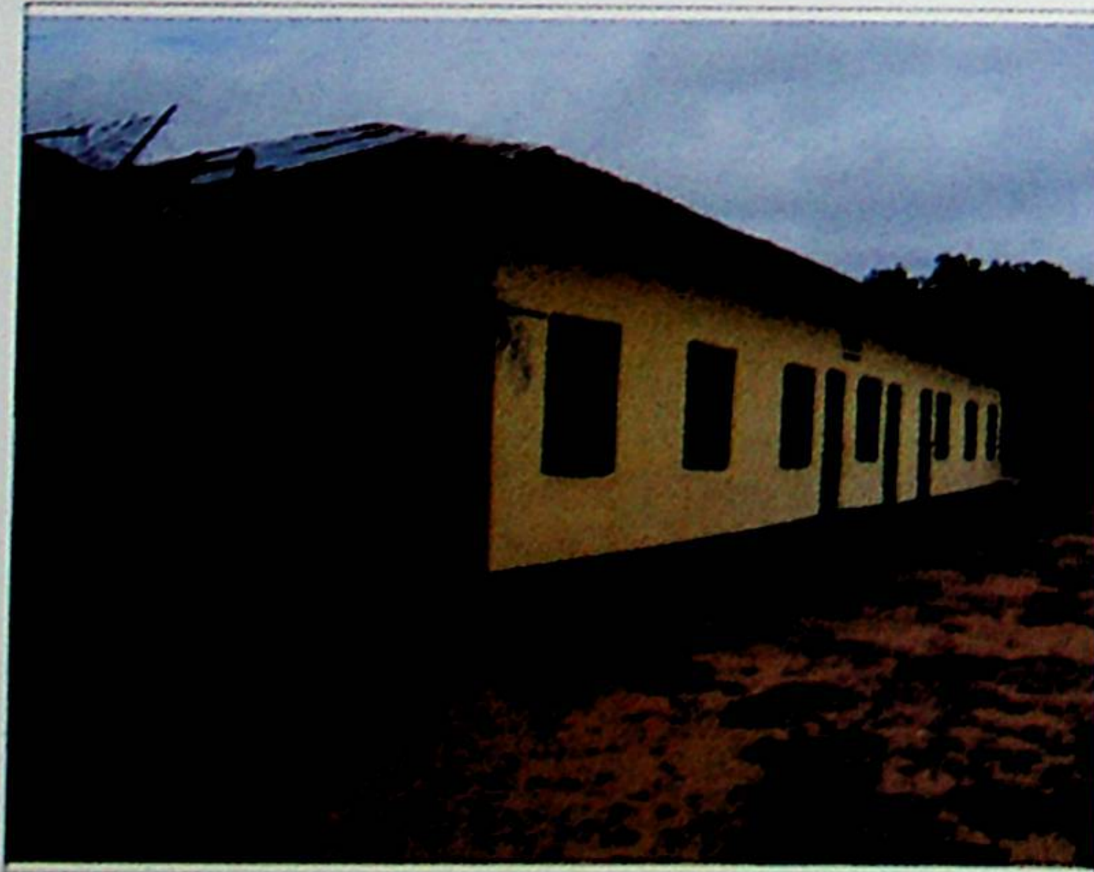
Renovation of One Block of 2 Classrooms & Office at Busu in Busu Ward
