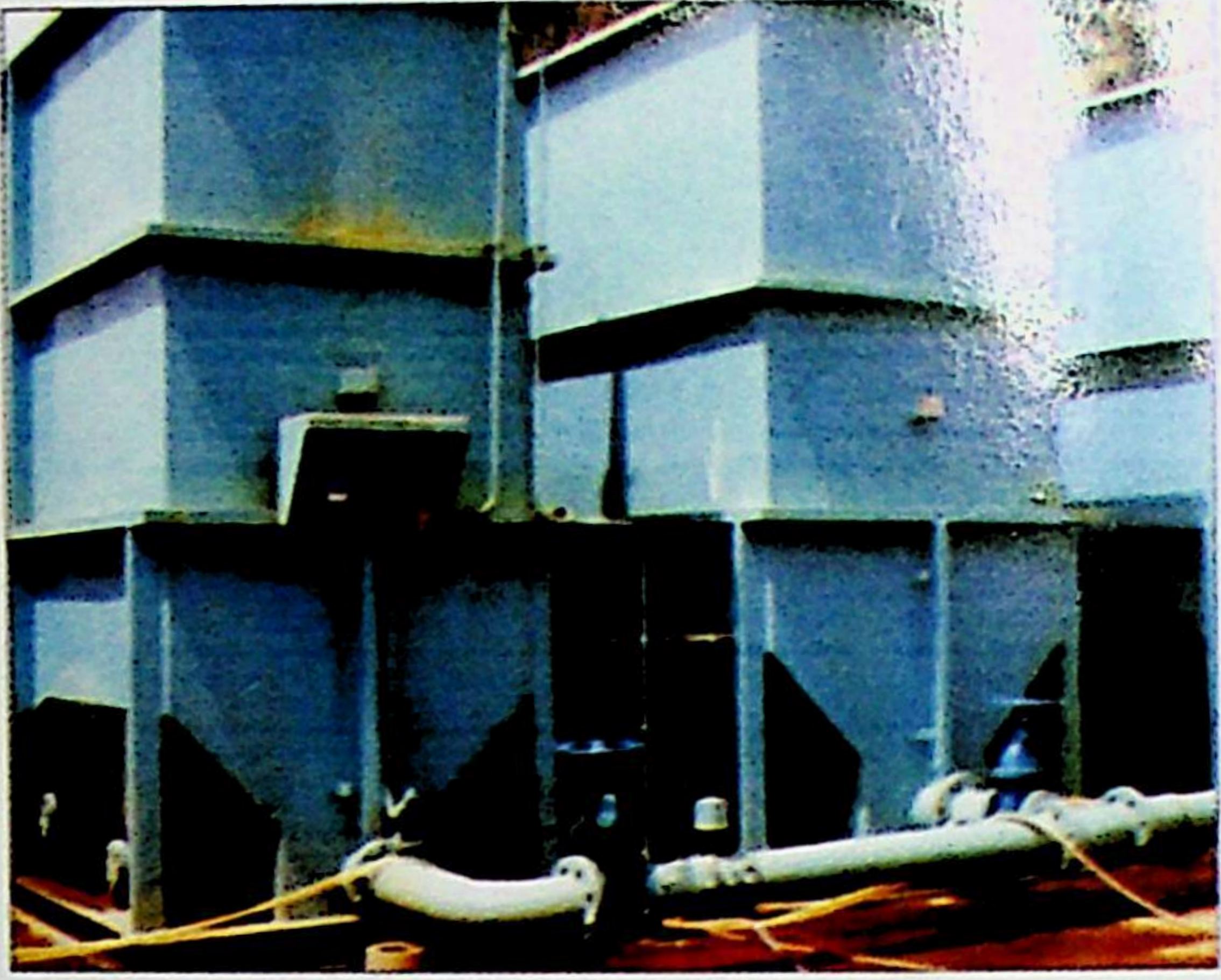
Bosso water treatment tank
