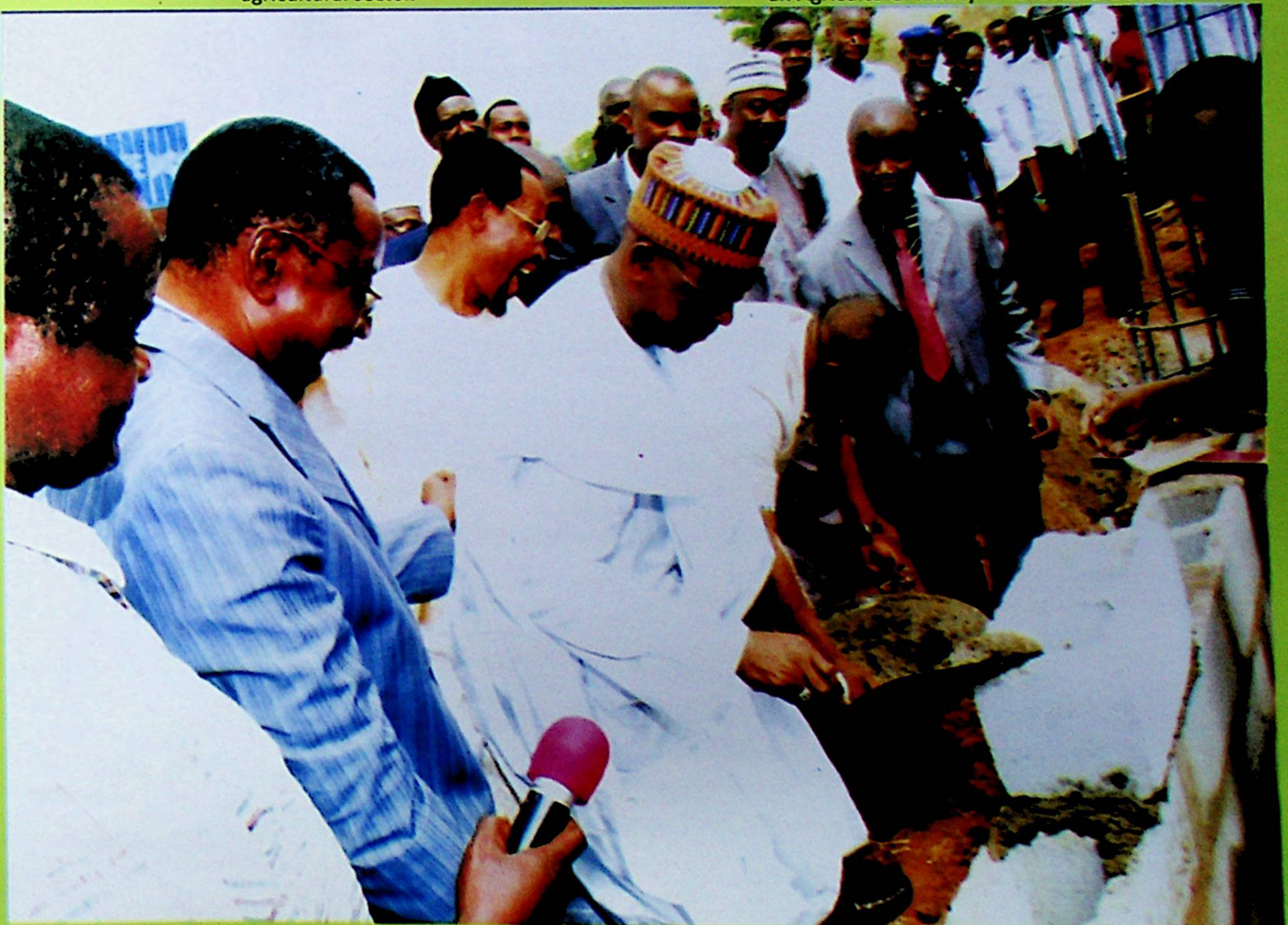
Governor Idris Wada laying the foundation stone for an Ultra Modern Lecture Theatre at Kogi State Polytechnic, Lokoja
