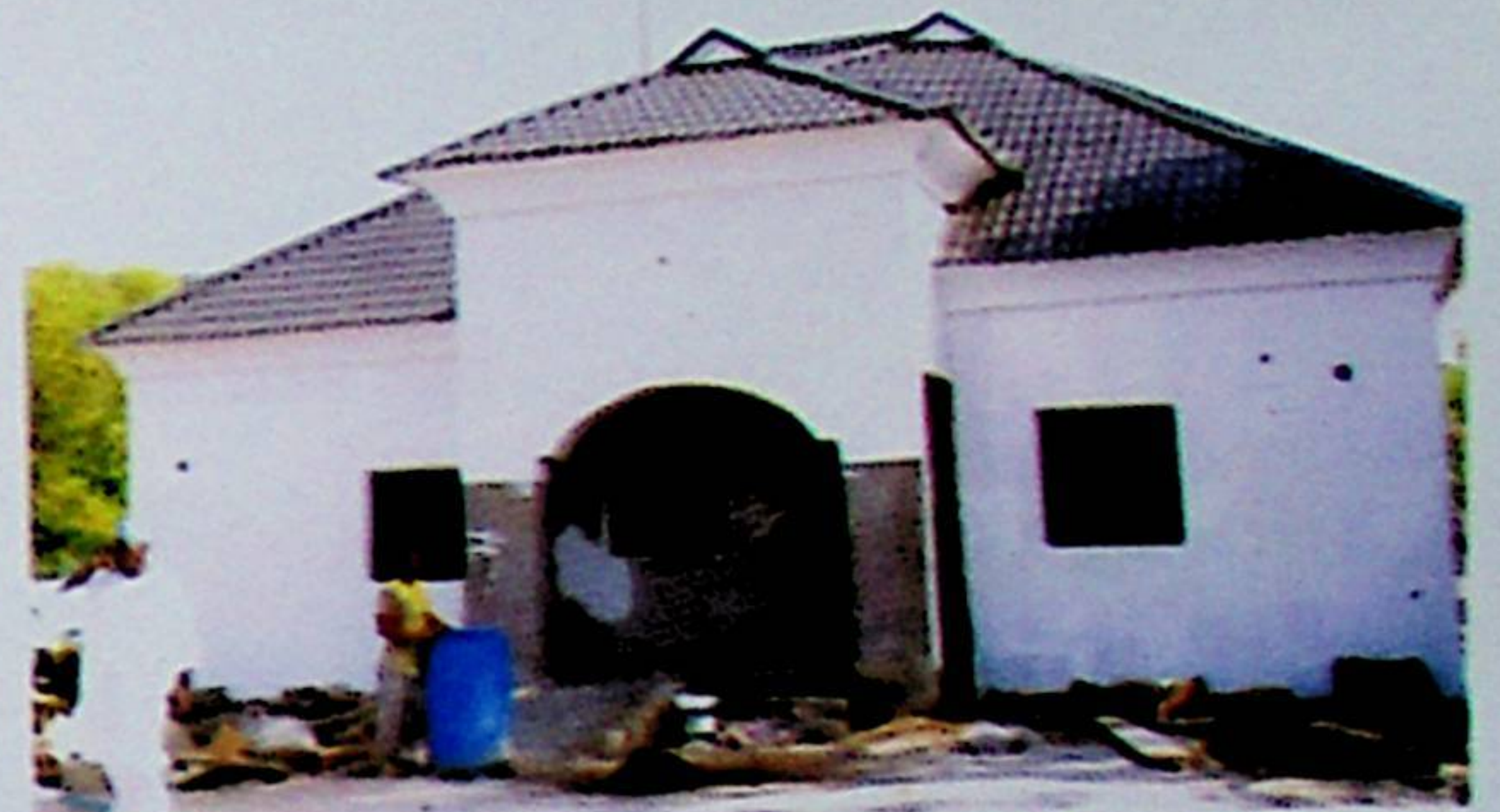
Work in progress on the New Government House Clinic being built by the Wada Administration.
