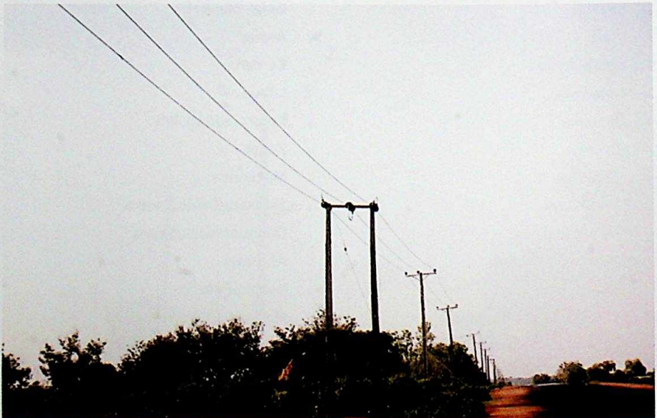
Electrification projects: solar (above) and the PHCN-powered ( below)
