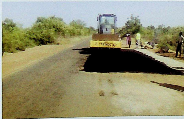
PRIMING AND ASPHALTIC CONCRETE RESEALING OF THE FAILED SECTION ON GWARAM-BASIRKA ROAD
