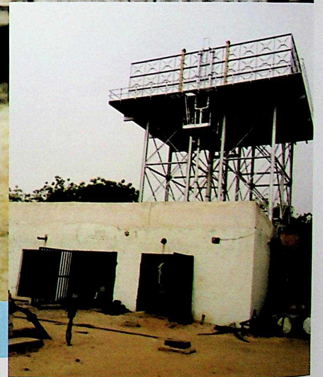
REHABILITATED GENERATOR ROOM AND 200M 3 OVERHEAD TANK AT HADEJIA MAIN PUMP HOUSE
