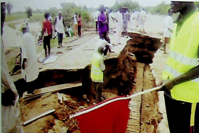
COMMISSIONER OF WORKS INSPECTING A SECTION OF GWARAM-BASIRKA ROAD AFFECTED BY FLOOD
