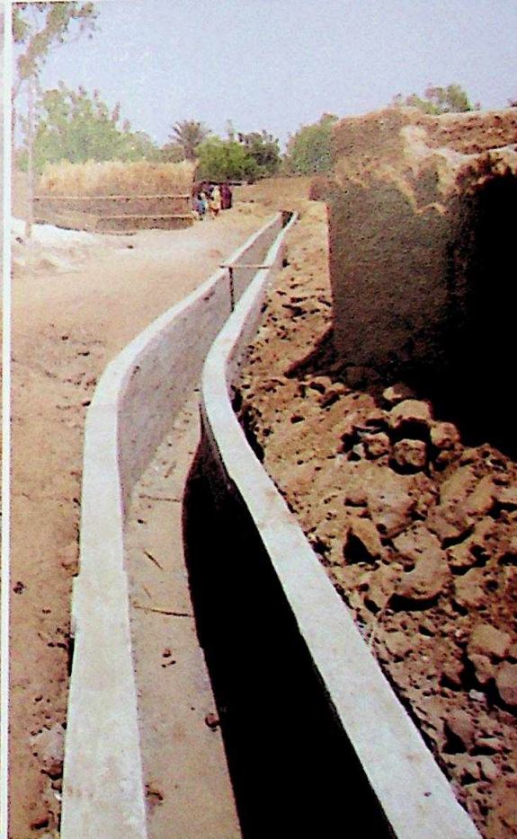
CONSTRUCTION OF DRAINAGES AND CULVERTS AT CHAMO TOWN, DUTSE LOCAL GOVERNMENT AREA
