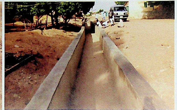
CONSTRUCTION OF DRAINAGES AND CULVERTS AT SAGU TOWN, BUJI LOCAL GOVERNMENT AREA
