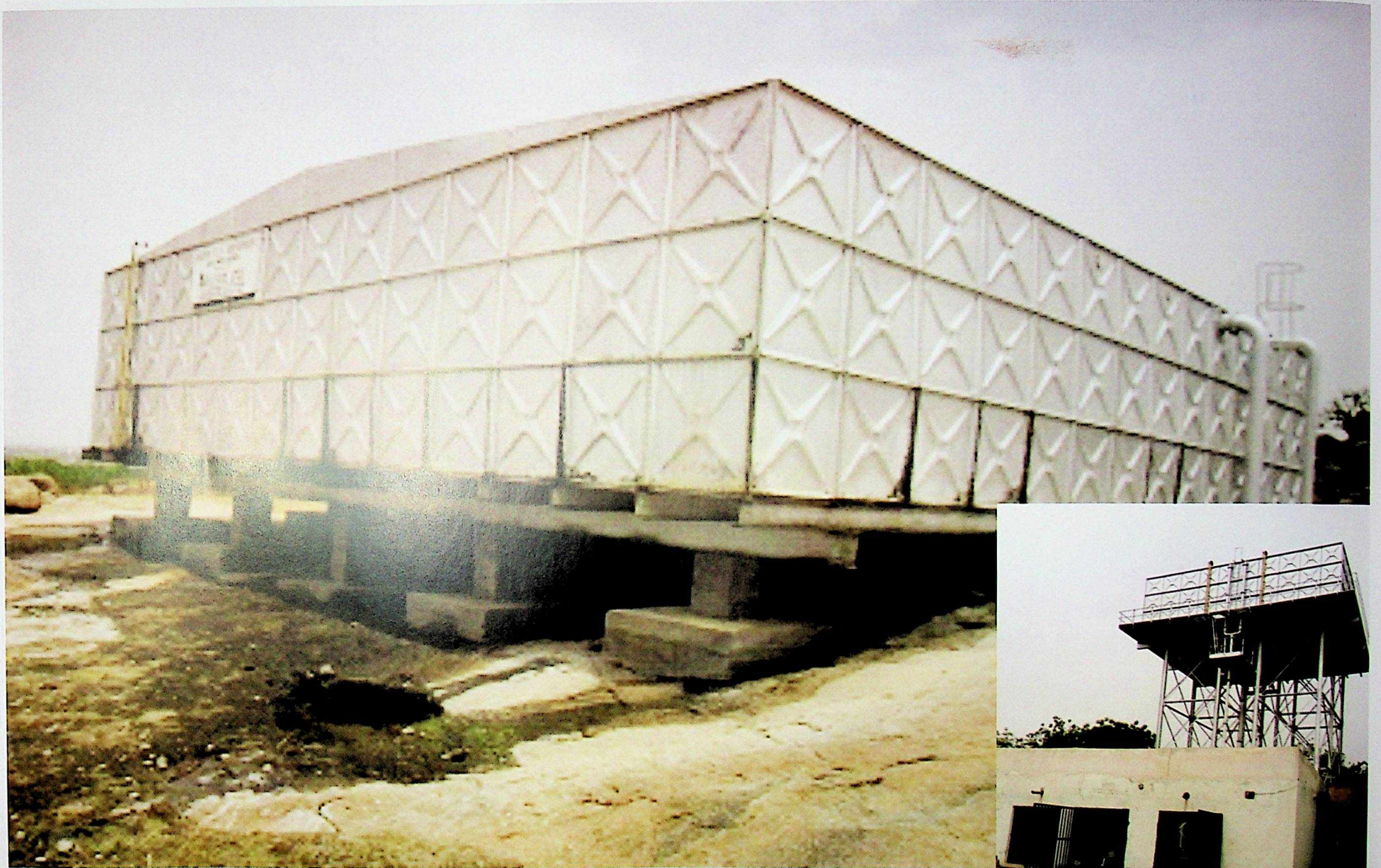
1 MILLION M 3 CAPACITY HILLTOP SURFACE TANK, ALONG KIYAWA ROAD DUTSE AFTER REHABILITATION
