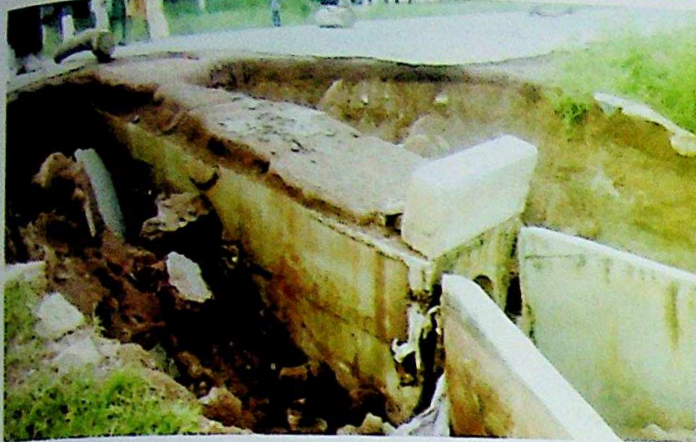
FAILED SECTION OF GADAMA CULVERTS (NO.1) ON GWARAM-FAGAM ROAD
