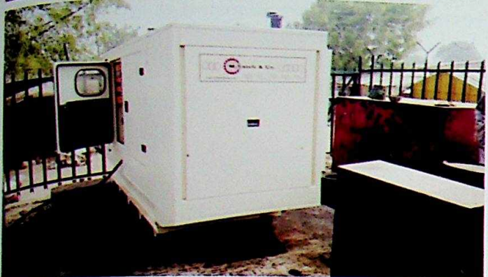
NEW 100 KVA GENSET AT KIYAWA MOSQUE
