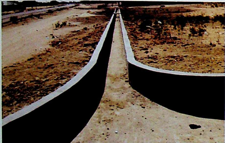
CONSTRUCTION OF DRAINAGES AND CULVERTS AT ASHURAN CHIROMA TOWN, KAFIN HAUSA LOCAL GOVERNMENT AREA
