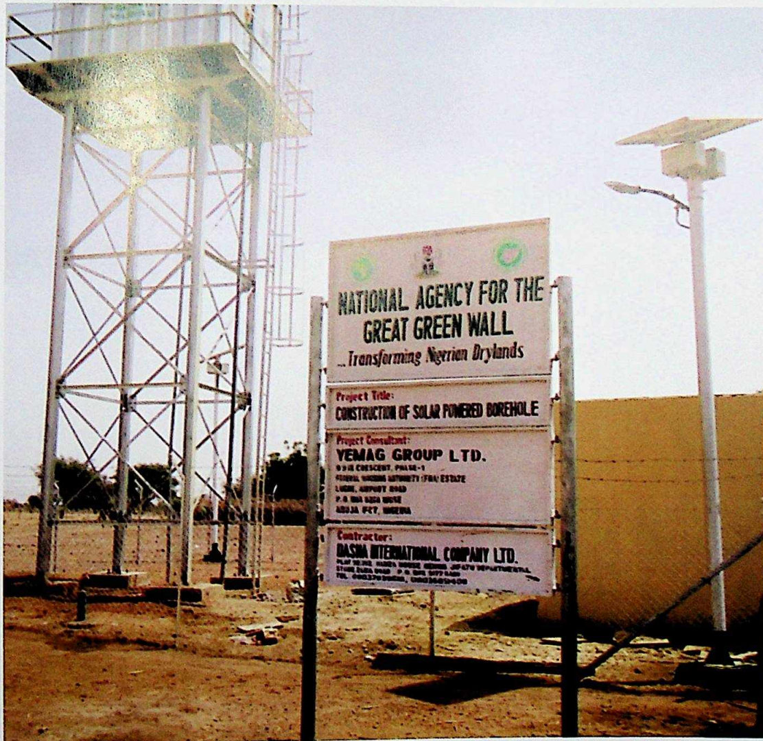
Solar borehole at Great Green Wall project site, Takure, Sule Tankarkar LGA
