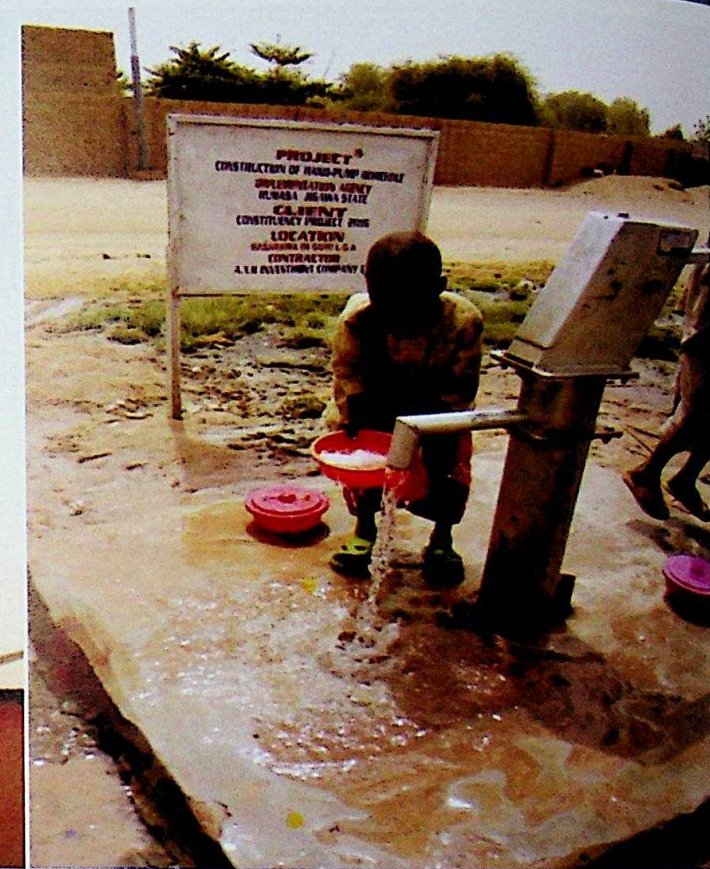
One of the newly constructed hand pump borehole in Nasarawa Guri LGA
