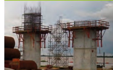
Early Works III, 2nd Niger Bridge, facilitating the movement of goods and services through increased road network.
