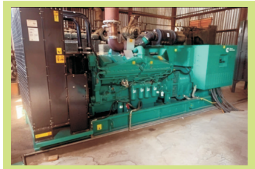
INSTALLED PANELS AND GENERATOR AT BIDA WATER WORKS
