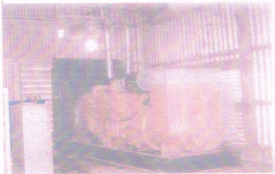
NEWLY GEN. SET OF (1000 KVA) INSTALLED AT CHANCHAGA WATER WORKS
