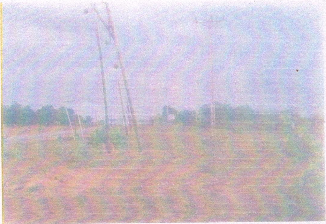
REPLACEMENT OF WOODEN ELECTRICAL POLES WITH CONCRETE POLES FROM CITY GATE TO CHANCHAGA WATER WORKS
