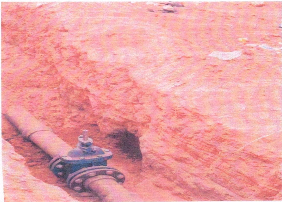
A 6" INSTALLED SLUICE VALVE
