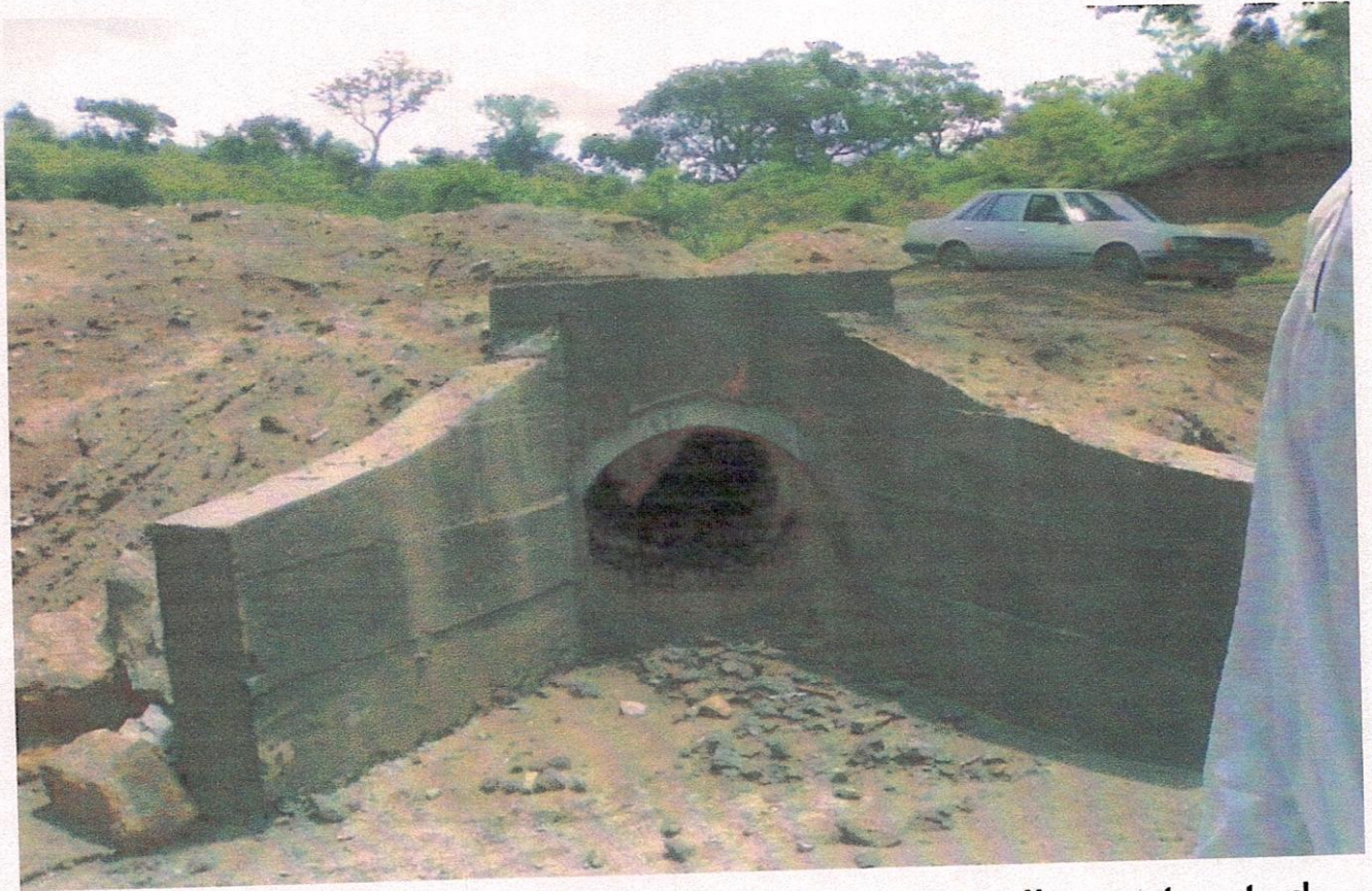
Pictures showing one cell and two cell constructed culvert along access road to dam site
