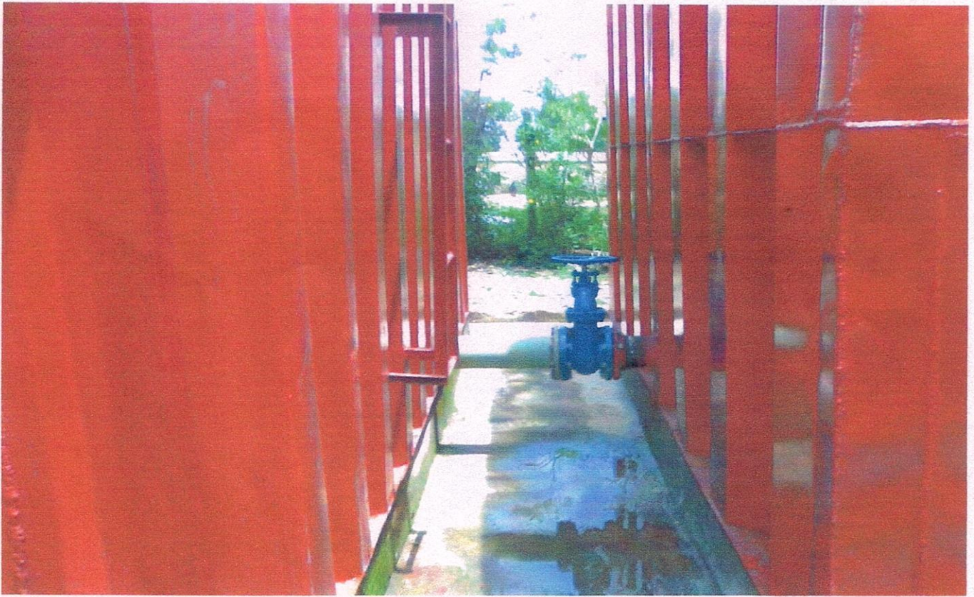
Picture showing interconnection of two clear water tanks
