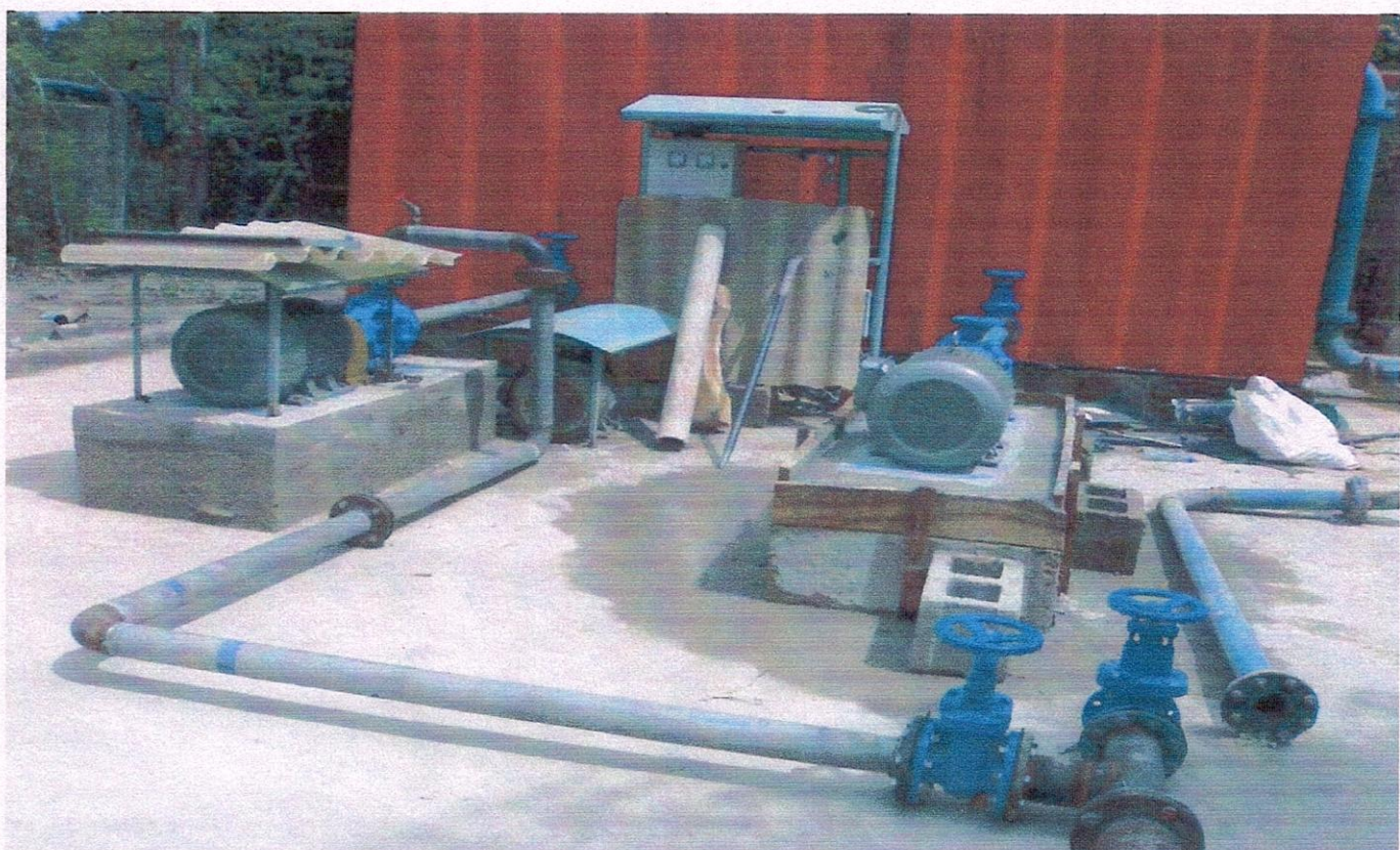
Picture showing the two installed 50hp high lift pumps supplied
