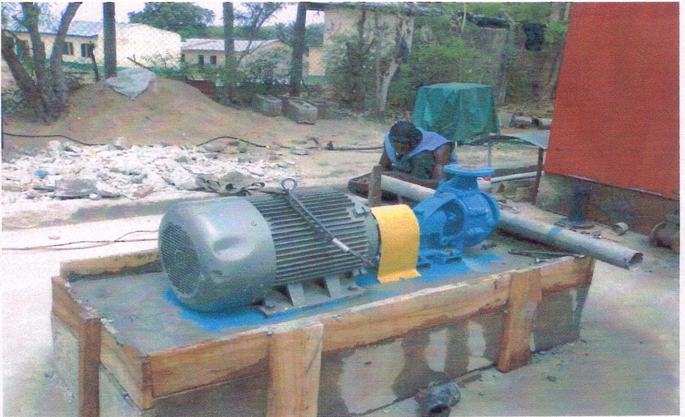
Picture showing the installation of 50hp high lift pump supplied
