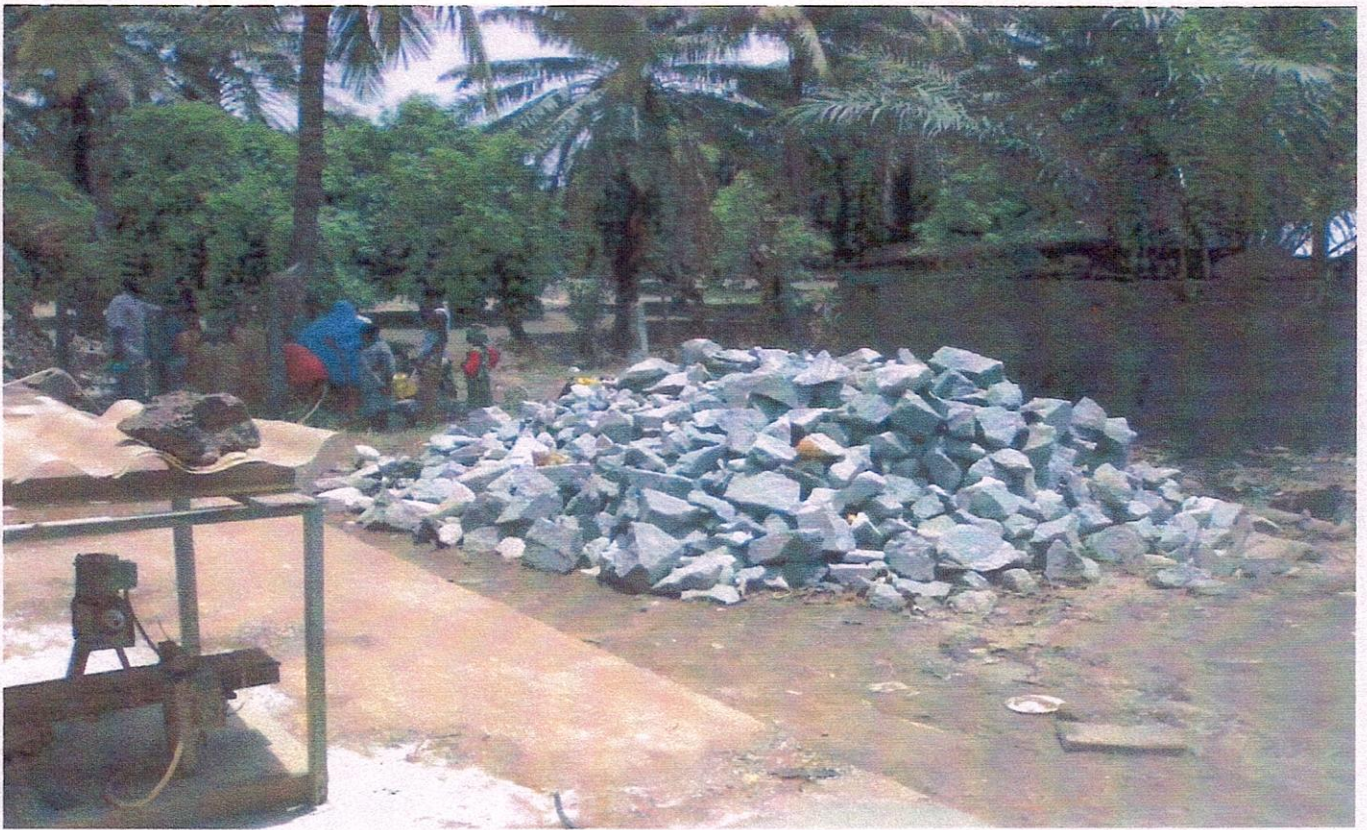
Picture showing hard core filling to enable access for mounting of the two packaged water treatment plants
