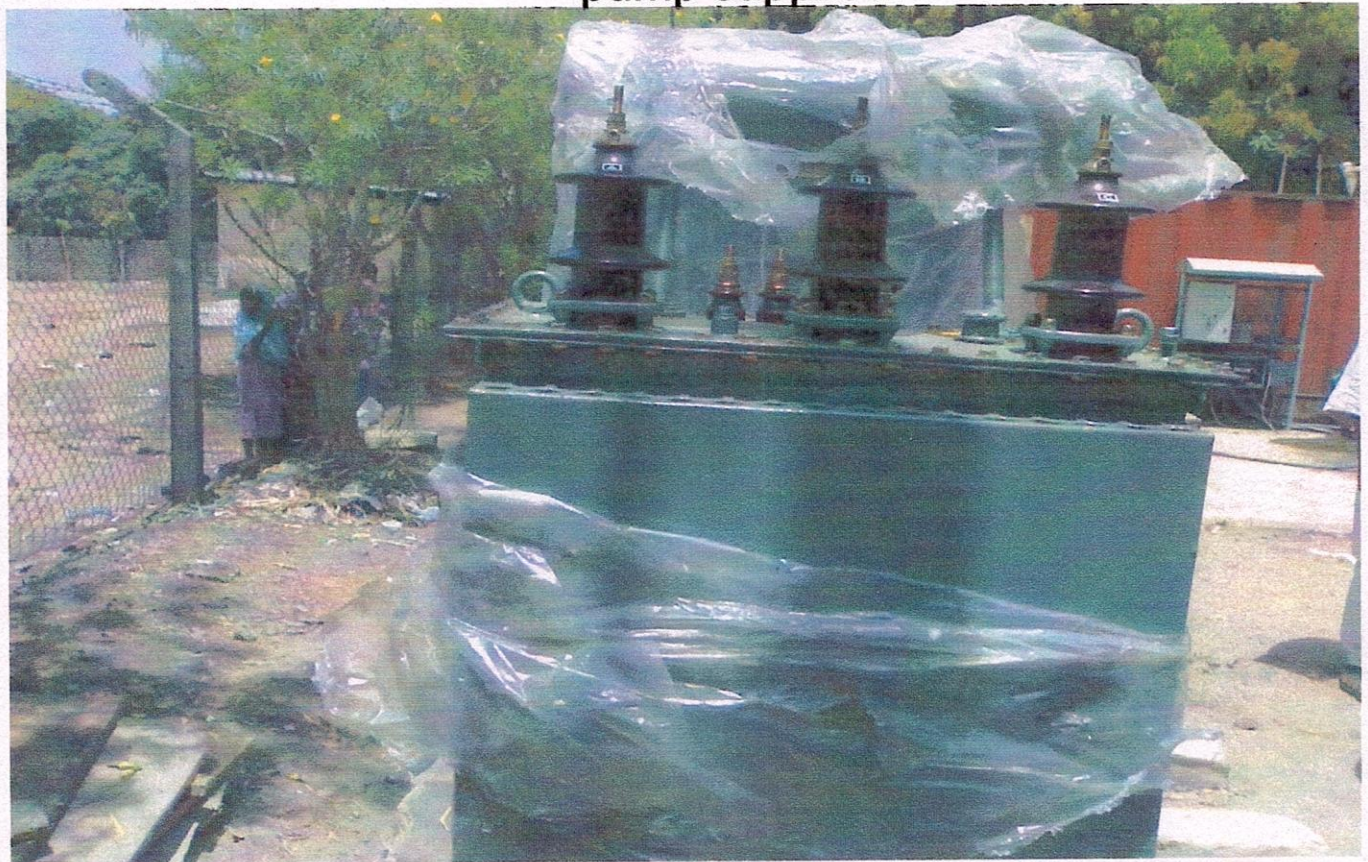
Picture showing 200kva transformer supplied
