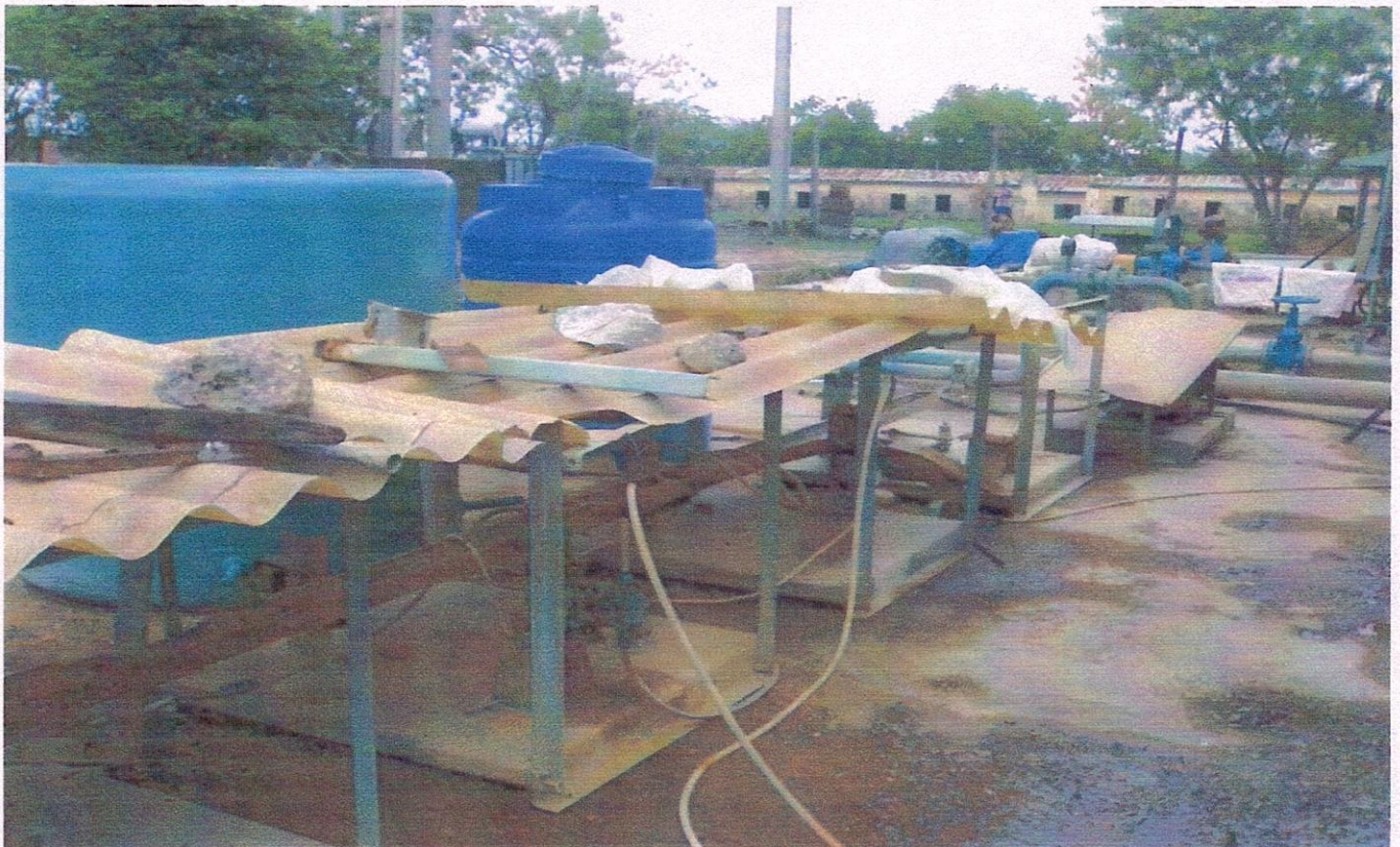
Picture showing replaced chemical dosing pumps
