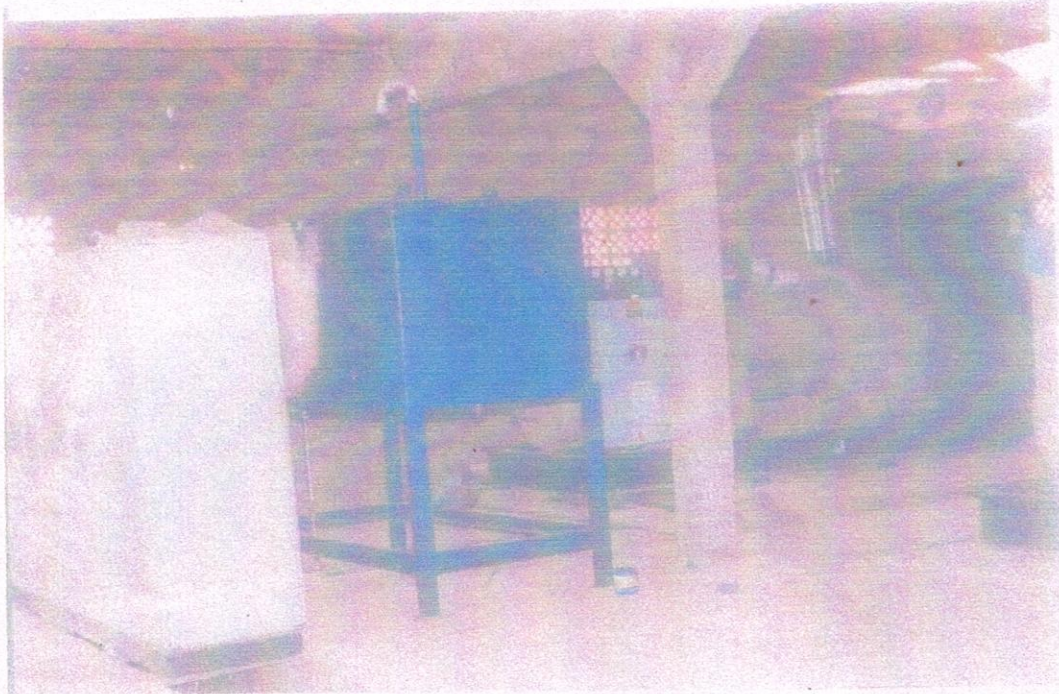
NEW GEN SET OF (1000 KVA) INSTALLED AT CHANCHAGA WATER WORKS
