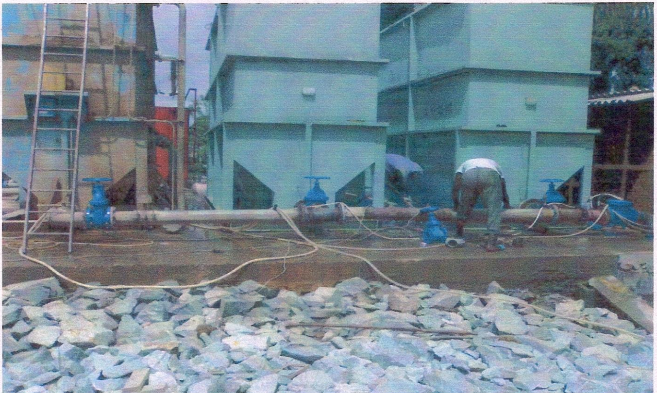
Picture showing the two installed packaged water treatment plants
