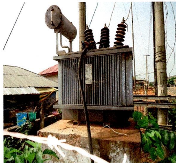
Irepodun LG-200KVA 33/0.415KV MINEL TRAF0 Transformer, S.N. 118312 at Esure Ekiti Ogbon Oba, Araromi-Ekiti.
