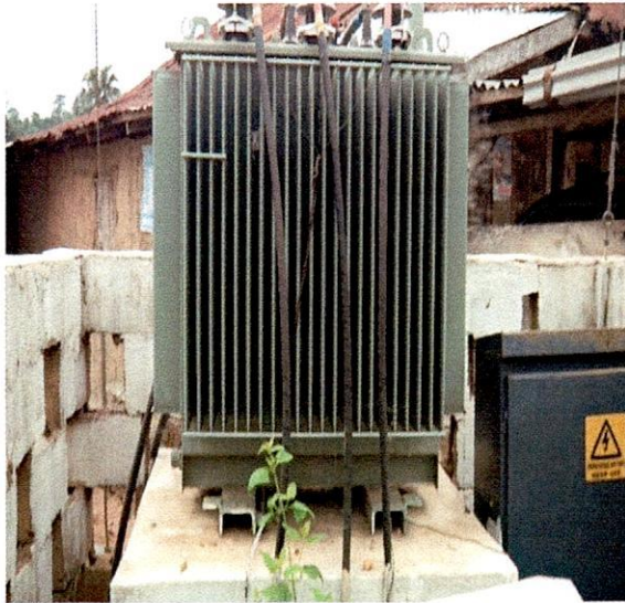
Ise-Orun LG-300KVA 11/0.415KV ABB Transformer, S.N.1LPL433057. Beside St. Paul School Ajegunle-Ekiti
