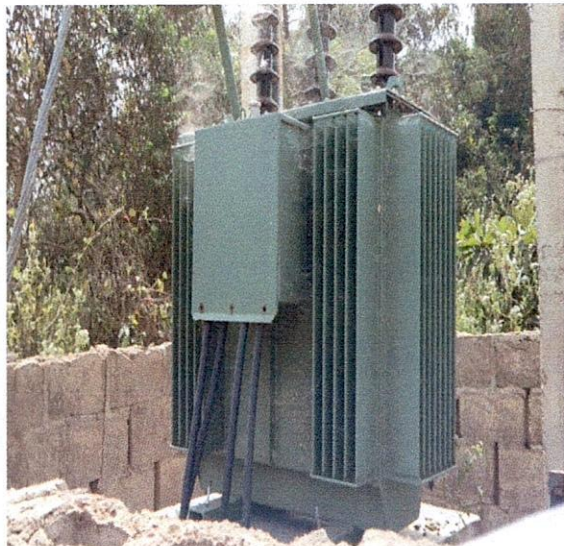
Ileje-Meje LG-300KVA 33/0.415KV Koncar Transformer, S.N.590785 at Iludun Ayo Village.
