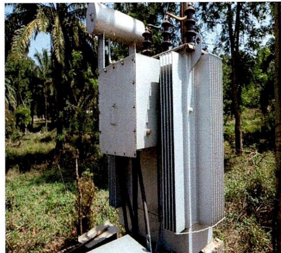
Moba LG-500KVA 33/0.415KV Emo-Ohrid Transformer, S.N.34845 Beside Adebisi Filling Station, Otun Ekiti.
