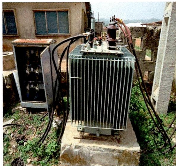
Irepodun LG-300KVA 33/0.415KV John holt Company Transformer, S.N., at Igedora Quarters, Araromi-Ekiti.
