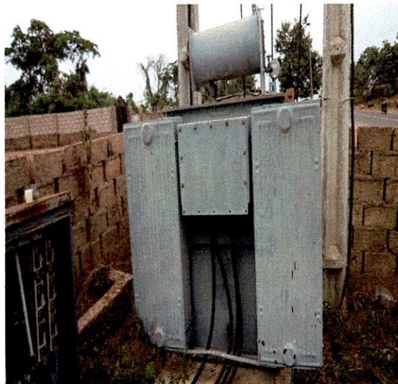
Ise-Orun LG-500KVA 11/0.415KV BRUSH Transformer, S.N.26520004. Opposite Omo-Oni Bus Stop, Orun-Ekiti
