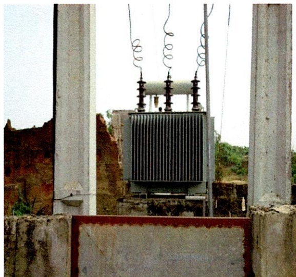
Irepodun LG-200KVA 33/0.415KV Zennaro Transformer, S.N..... Oluri Compound, Araromi Ekiti
