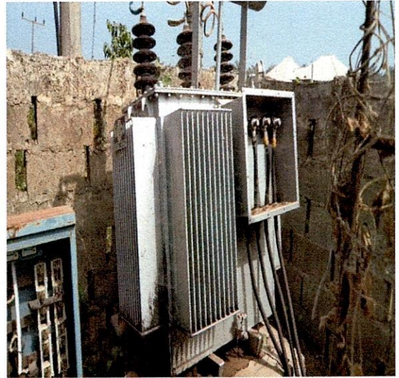
Ileje-Meje LG-500KVA 33/0.415KV Kotco Transformer, S.N.K140 Opposite Ijeshamodu Mordern Market, Ekiti.
