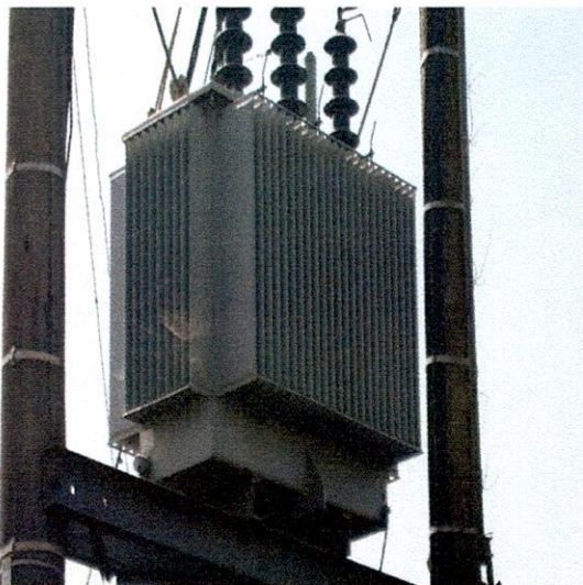
Ileje-Meje LG-KVA 33-0.415KV Transformer, S.N., Along Kwara State Road, Ijeshamodu.
