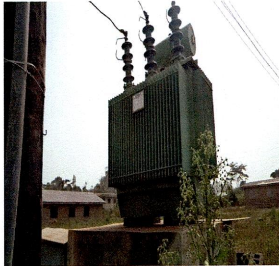
Moba LG-200KVA 33/0.415KV Koncar Transformer, S.N.6TBN200388 at Good Shepherd Catholic Church, Igogo-Ekiti
