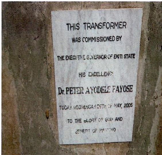
A plaque at Ileje-Meje LG-500KVA 33/0.415KV Kotco Transformer, S.N.K140 Opposite Ijeshamodu Mordern Market, Ekiti.
