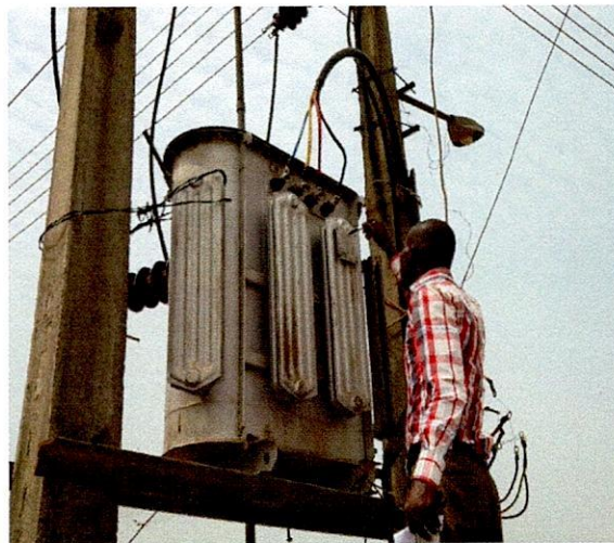
Irepodun LG-50KVA 33/0.415KV Minel Transformer, S.N. TP.7413.50 at Afin Junction, Irapora Ekiti
