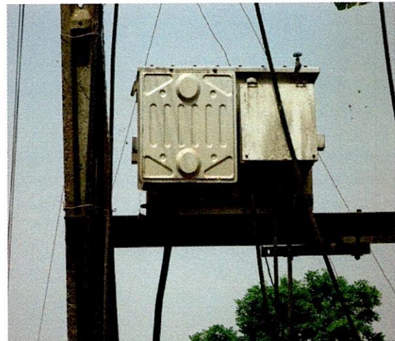
Irepodun LG-100KVA 33/0.415KV Transformer, S.N.... Opposite Eyemote Comprehensive High School, Araromi Ekiti
