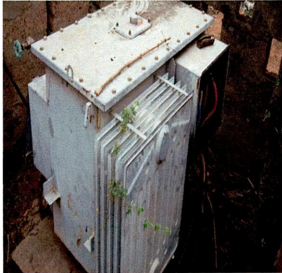
Ise-Orun LG-300KVA 33/0.415KV Mitsubishi Transformer, S.N.L31691006 at St. Stephen Anglican School, Erinwa, Ekiti
