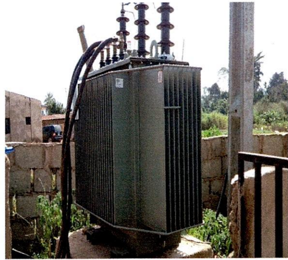
Moba LG-300KVA 33/0.415KV ABB Transformer, S.N. 1LPL463632 at The Apostolic Faith Church, Oke Owa Street, Igogo-Ekiti.
