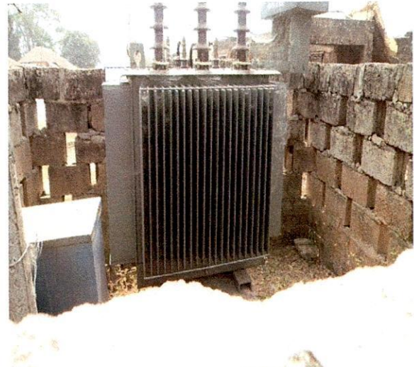
Oye LG- 300KVA 33/0.415KV Elsewedy Electric Transformer S.N. 1003000800 Opposite St. Paul Anglican Church, Ijelu Ekiti.
