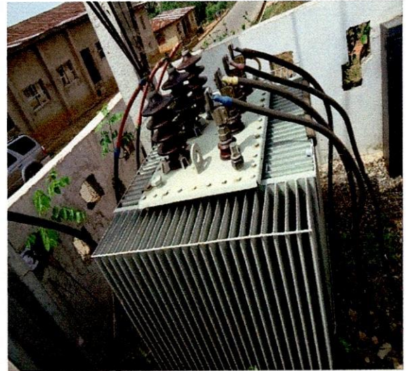
Irepodun LG-500KVA 33/0.415KV Elvim Transformer, S.N.RV.2008.W.523.3048 Behind C.A.C Oke Iye Awo Road, Araromi Ekiti
