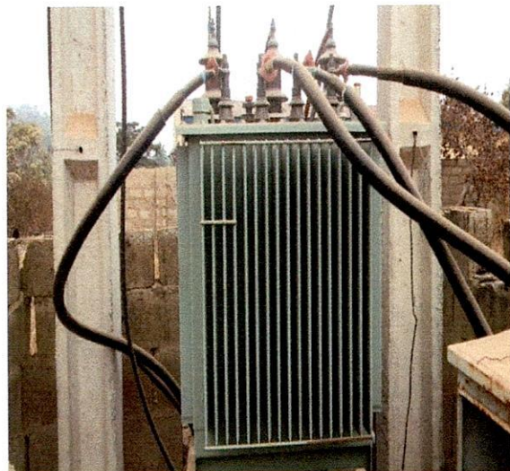
Oye LG- 300KVA 33/0.415KV ABB Transformer S.N. 364014 at Irare Estate.
