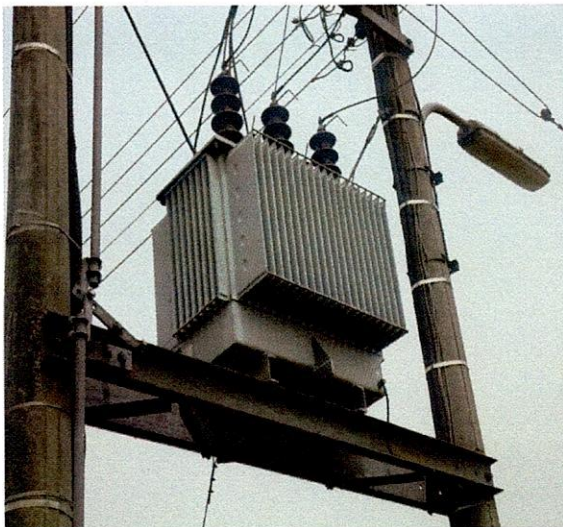
Irepodun LG-200KVA 33/0.415KV Transformer, S.N...at Oke Orun Junction, Igbemo, Araromi-Ekiti.
