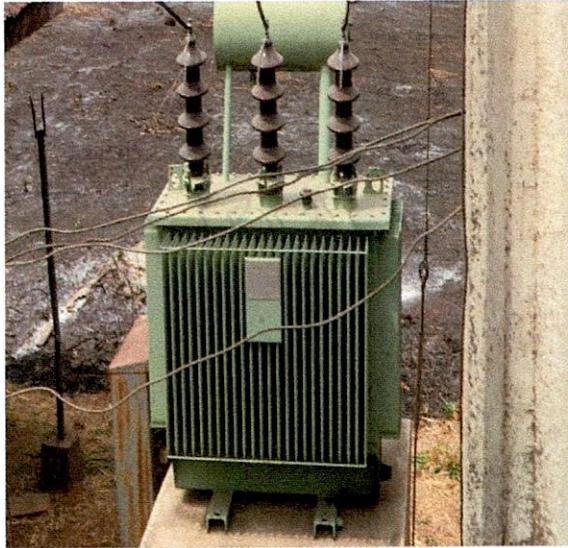
Oye LG- 300KVA 33/0.415KV Transformer S.N., at Ogunlade Sawmill, Oye
