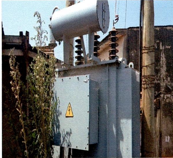
Moba LG-500KVA 33/0.415KV JSC Ukrelectroapparat Transformer, S.N. 435757 Beside Co-operative Hall, Odo-Oja, Otun-Ekiti.
