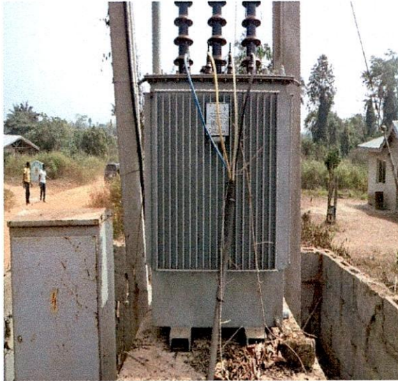
Ileje-Meje LG-200KVA 33/0.415KVABB Transformer, S.N.DT5612406 Opposite Community Primary School, Ipere-Ekiti.
