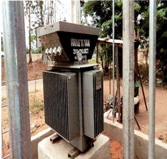
Ise-Orun LG-300KVA 11/0.415KV Elsewedy Transformer, S.N.1003000510 at the General Hospital, Ise-Ekiti
