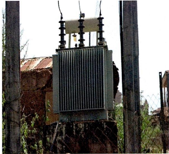
Moba LG-200KVA 33/0.415KV Elettromeccanica Transformer, S.N. 18041 at Customary Court Junction, Erinmope-Ekiti.
