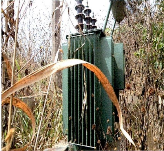
Ileje-Meje LG-300KVA 33/0.415KV Konkar Transformer, Along Ipere Road, Iye-Ekiti.
