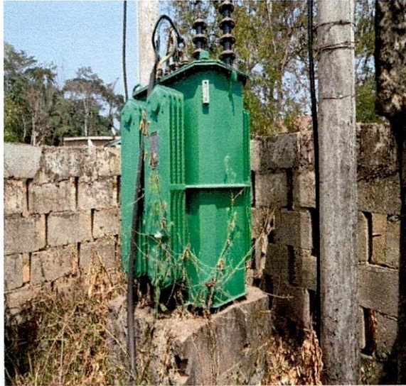
Ileje-Meje LG-200KVA 33/0.415KV Bi Bong Transformer, S.N.030059 Opposite St. Boniface Catholic Nursery & Primary School, Iye-Ekiti.
