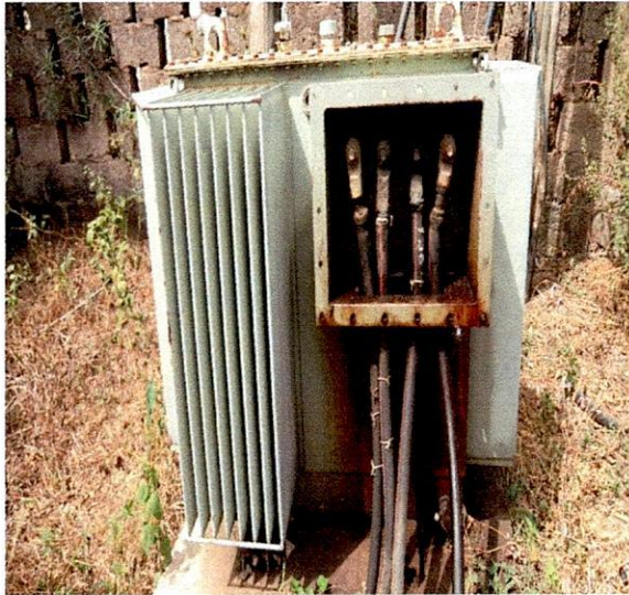
Ise-Orun LG-200KVA 11/0.415KV Trafo Union Transformer, S.N.21820539. at Ise-Orun LG Secretariat, Ekiti
