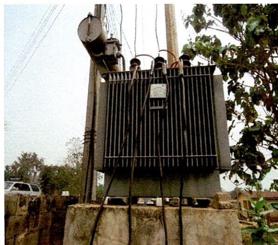
Irepodun LG-300KVA 33/0.415KV ABB ELEKTRIK Transformer, S.N.DT.40209.06 at Surulere Street, Opposite Living Faith, Iworoko, Araromi-Ekiti.
