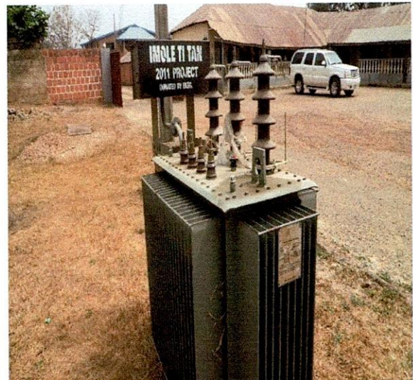
Oye LG- 300KVA 33/0.415KV Elsewedy Electric Transformer S.N. 1003000430 at Onire Palace, Ire Ekiti
