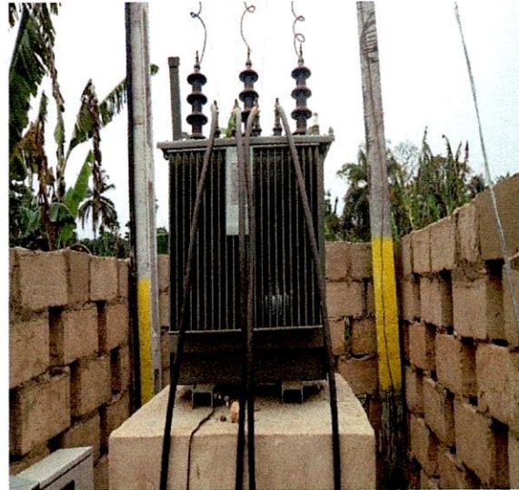
Ise-Orun LG-200KVA 33/0.415KV ABB Transformer, S.N.1LPL465765 at Aba Ede, Ise-Orun.
