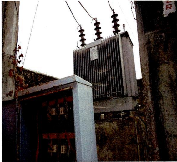
Irepodun LG - 200KVA 33/0.415KV Emo-Ohrd Transformer, S.N. ETBK200.35 Opposite Palace Araromi, Araromi Ekiti
