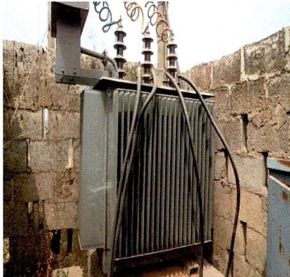
Oye LG- 300KVA 33/0.415KV Elsewedy Electric Transformer S.N. 1003000434 Opposite Ayede Grammar School, Ayede.
