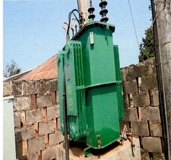
Ileje-Meje LG-200KVA 33/0.415KVBi Bong Transformer, S.N.K030064431 Beside Market Sqaure, Ewu-Ekiti.
