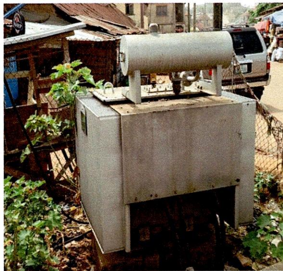
Irepodun LG-200KVA 33/0.415KV, S.N..... Ijoka Street, Igede, Araromi -Ekiti
