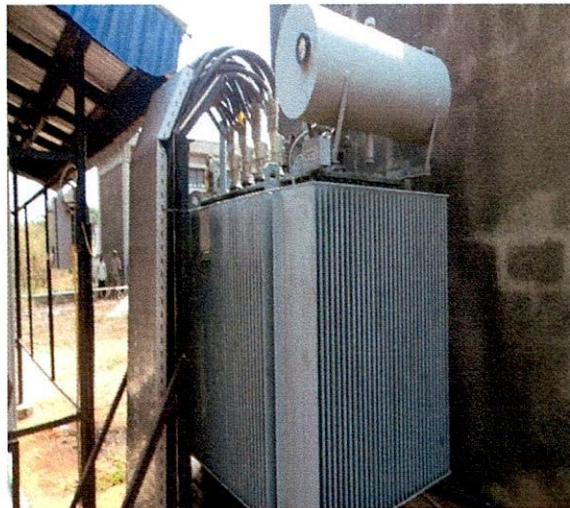
Moba LG-2500KVA 33/0.415KV AREVA Transformer, S.N.39049556 Ekiti State, Water Corporation V, Ero Dam, Ikun-Ekiti
