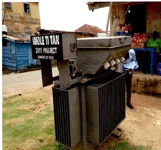
Irepodun LG-200KVA 33/0.415KV Minel Trafo Transformer, S.N.107550 at Eyio Ekiti Opposite C.A.C Oke Agbara, Araromi Ekiti
