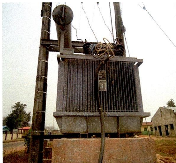
Irepodun LG-200KVA 33/0.415KV MINEL Transformer, S.N.118313 Opposite Are Community Health Center, Araromi-Ekiti.,
