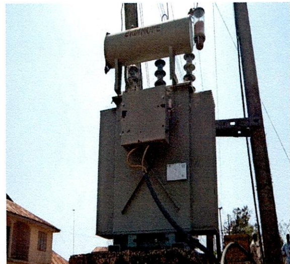
Moba LG-300KVA 33/0.415KV Pauwels Transformer, S.N. 99N-1824 Beside St. John, Iloye Street, Erinmope-Ekiti.
