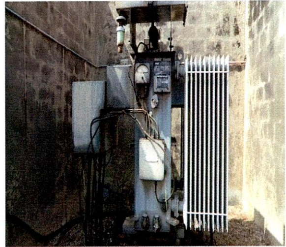
Moba LG-630KVA 33/0.415KV GEC Transformer, S.N.813681 Ekiti State Water Corporation II, Ero Dam, Ikun-Ekiti.
