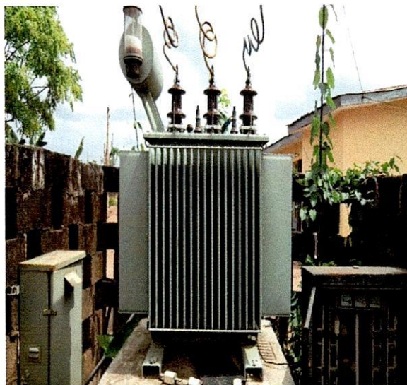
Ise-Orun LG-300KVA 11/0.415KV Siemens Transformer, S.N.C158484 at Kajola, Temidire, Ekiti
