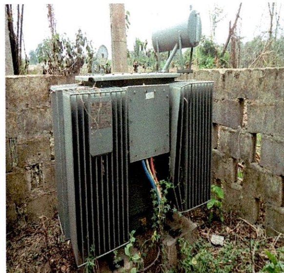
Ise-Orun LG-300KVA 11/0.415KV Elprom Trafo Transformer, S.N.141431 at Oge Street, Ise-Ekiti
