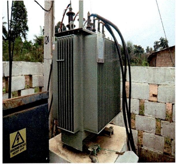
Ise-Orun LG-300KVA 11/0.415KV ABB Transformer, S.N.1LPL433060. In front of CAC Ajegunle-Ekiti
