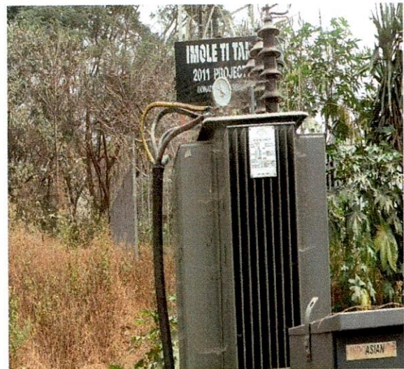
Oye LG- 300KVA 33/0.415KV Elsewedy Electric Transformer S.N. 1003000424 Opposite Oke Alafia Junction, Ayede Ekiti.
