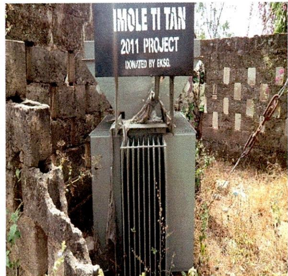
Ise-Orun LG-500KVA 11/0.415KV Elsewedy Transformer, S.N.1005000455 along Ise-Orun LG Secretariat Road, Ekiti
