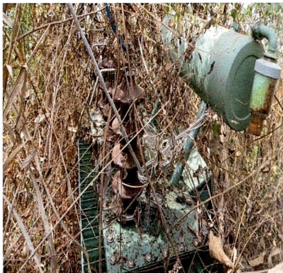
Ileje-Meje LG-300KVA 33/0.415KV Koncar Transformer, S.N. at Iludun Command Junior High School, Isan Road.
