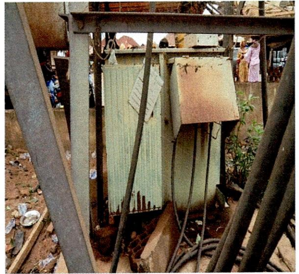
Ise-Orun LG-300KVA 11/0.415KV BREDA Transformer, S.N.1863805. Beside Post Office, Orin Ekiti, Ekiti
