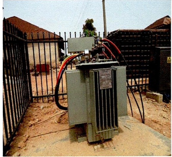
Irepodun LG-300KVA 33/0.415KV Elsewedy Transformer, S.N..., Opposite Baptist Primary School, Araromi Ekiti
