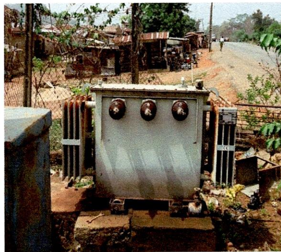
Irepodun LG-300KVA 33/0.415KV ABB Transformer, S.N..... Opposite Health Post, Ilawe Road, Araromi Ekiti
