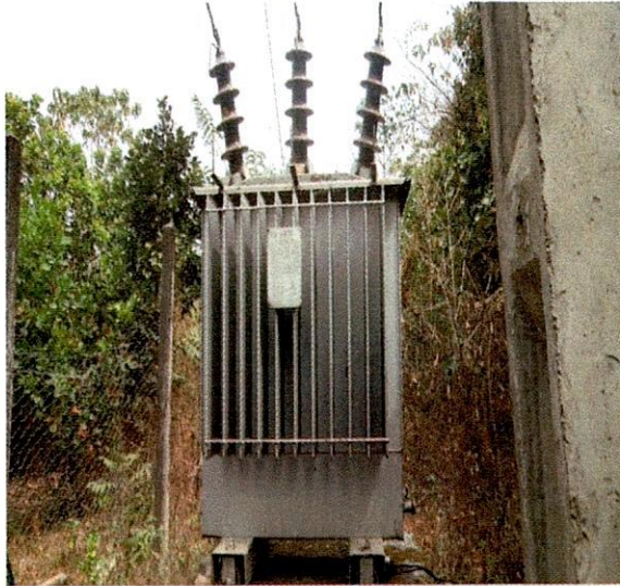
Oye LG- 100KVA 33/0.415KV Emo-Ohrid Transformer S.N. 33707 at Water Booster Station, Ilupeju.
