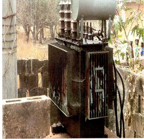
Oye LG- 300KVA 33/0.415KV Siemens Transformer S.N. 833193 along Ogere Industrial Estate, Ayede
