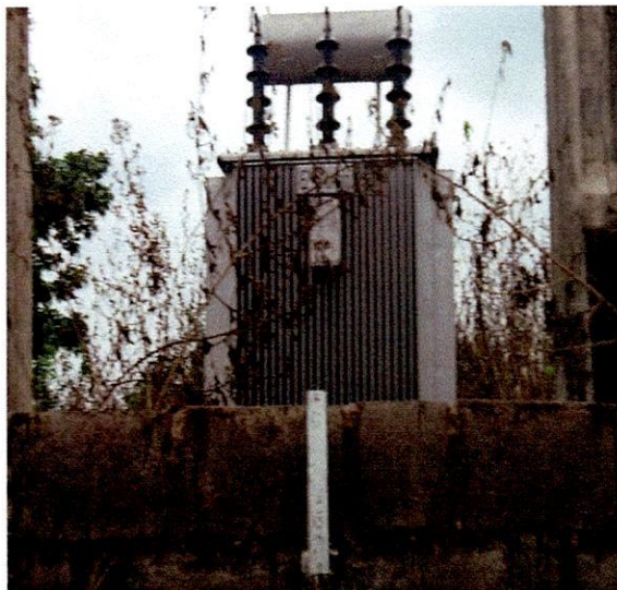
Ise-Orun LG-200KVA 33/0.415KV Emo-Ohrid Transformer, S.N.88420 at Egbese, Ise-Orun
