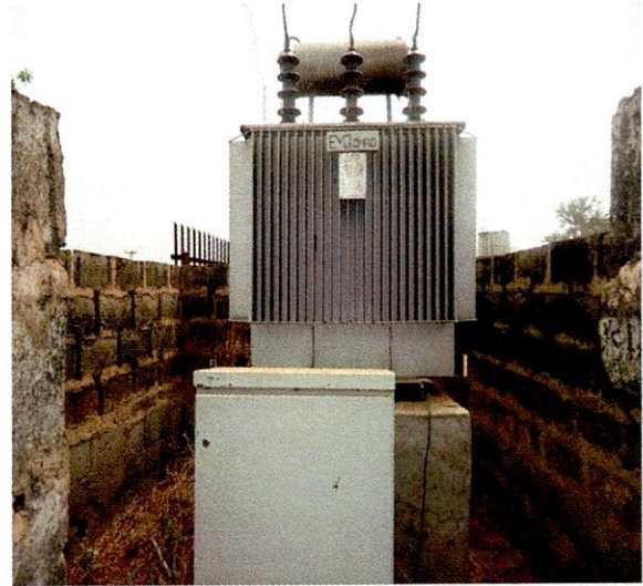
Irepodun LG-300KVA 33/0.415KV Emo-Ohrid Transformer, S.N.39450 at Roundabout, Afao, Araromi-Ekiti.
