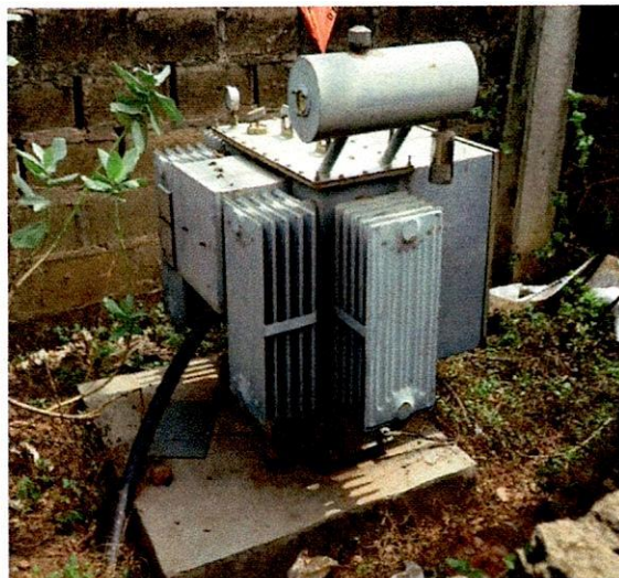
Irepodun LG-500KVA 33/0.415KV, S.N., Marter Christi Road, Ararom-Ekiti
