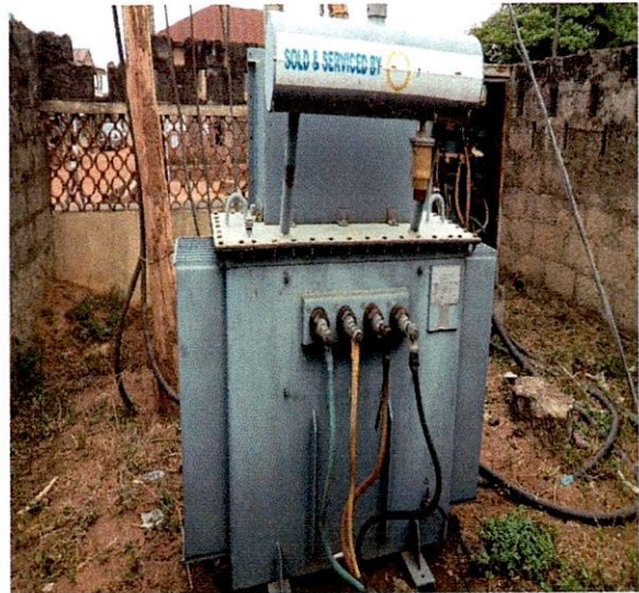
Ise-Orun LG-300KVA 11/0.415KV John Holt Transformer, S.N.500500 at St. Paul Anglican Church Oraye, Ekiti
