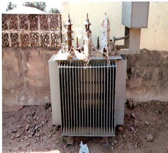
Moba LG-500KVA 33/0.415KV Else-wedy Transformer, S.N. 1003000338 at Kabiyesi Palace, Osan Ekiti.
