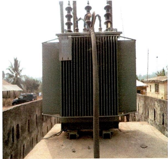
Oye LG- 300KVA 33/0.415KV ABB Transformer S.N. 1LPL359951 Imojo Rural Electrification, Imojo Ekiti.
