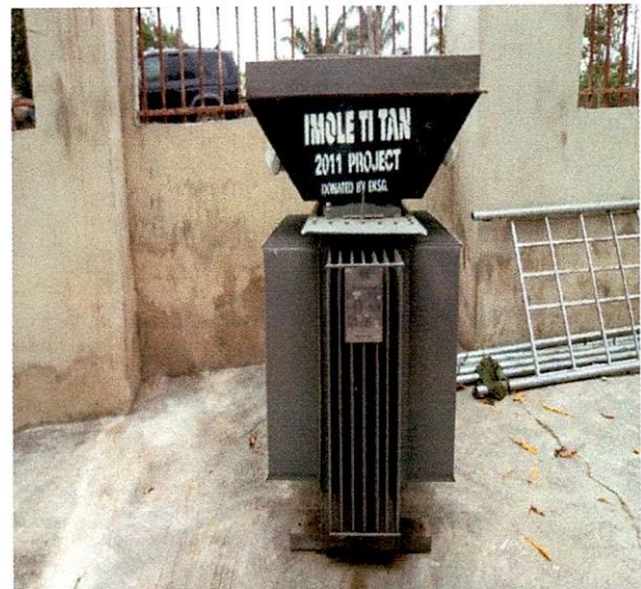
Ise-Orun LG-300KVA 33/0.415KV Elsewedy Transformer, S.N.1003000505. Olowuro Palace, Orun-Ekiti
