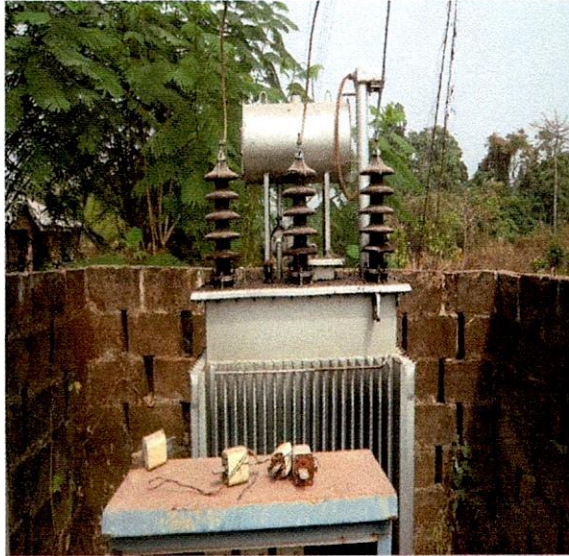
Oye LG- 300KVA 33/0.415KV Kotson Transformer S.N. 99878 Opposite Jagun Ajakaye, Isan Ekiti.
