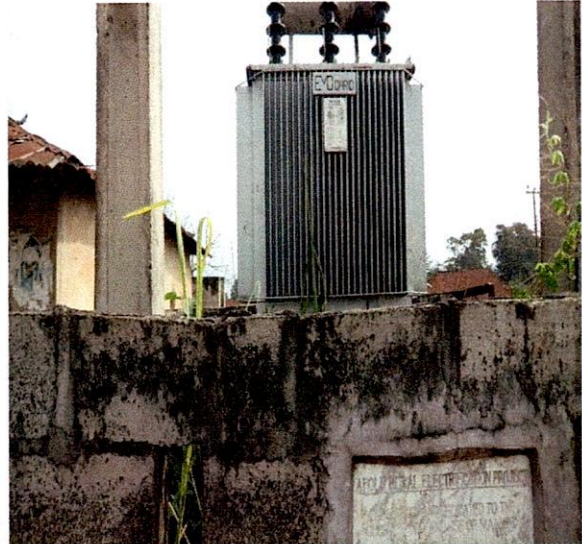
Ise-Orun LG-200KVA 33/0.415KV Emo-Ohrid Transformer, S.N.339201. Beside GOFAMINT Afolu, Ekiti
