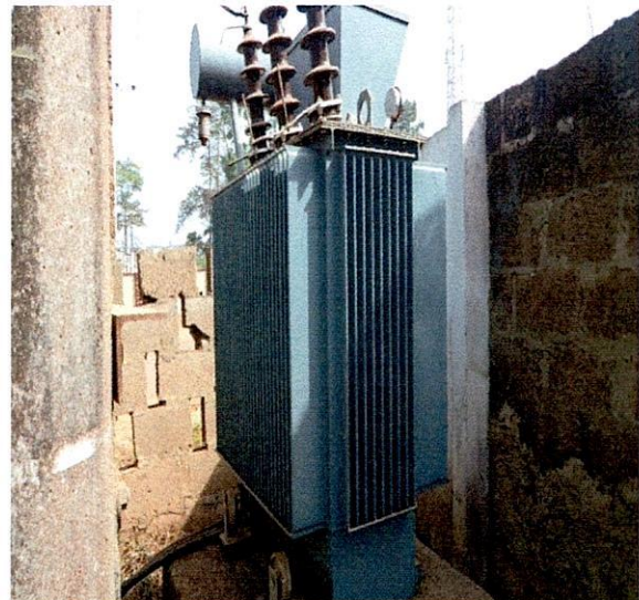
Ileje –Meje LG-500KVA 33/0.415KV Zennaro Transformer, S.N.49344 Opposite Palace, Iye-Ekiti.
