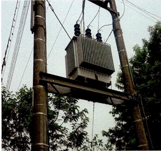
Irepodun LG-200KVA 33/0.415KV Transformer, S.N... at Ansaar-ud-deen Primary School, Araromi-Ekiti.
