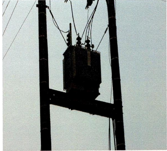
Oye LG- Siemens Transformer S.N. 33-0.415KV at Ijelu Road, Itapa-Ekiti.
