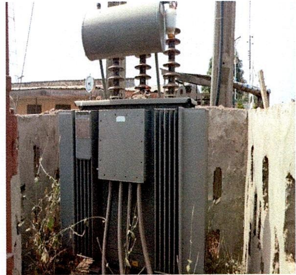
Ileje-Meje LG-300KVA 33/0.415KV Elprom Transformer, S.N.141177 at Eda- Oniyo 'T' Junction.
