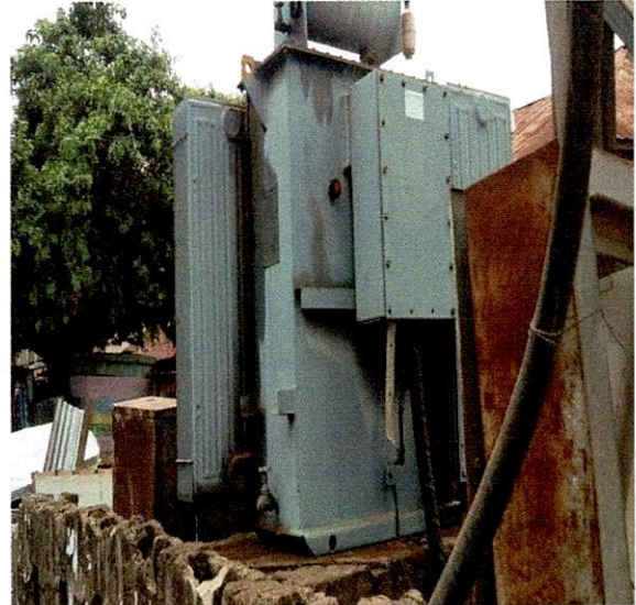
Ise-Orun LG-500KVA 11/0.415KV BRUSH Transformer, S.N... at Ojude Street, Orun Ekiti
