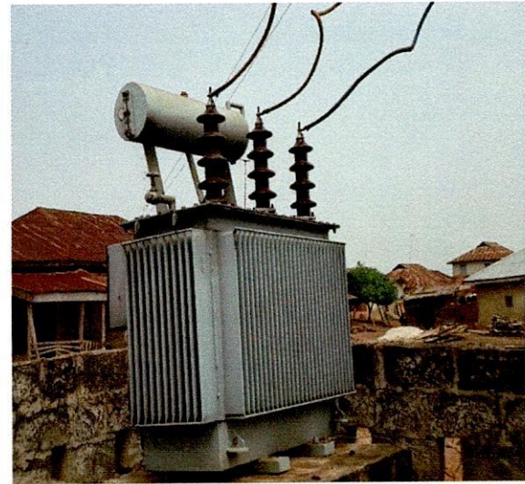
Irepodun LG-300KVA 33/0.415KV Marson's Transformer, S.N..., at St. Theresa's Junction, Araromi-Ekiti
