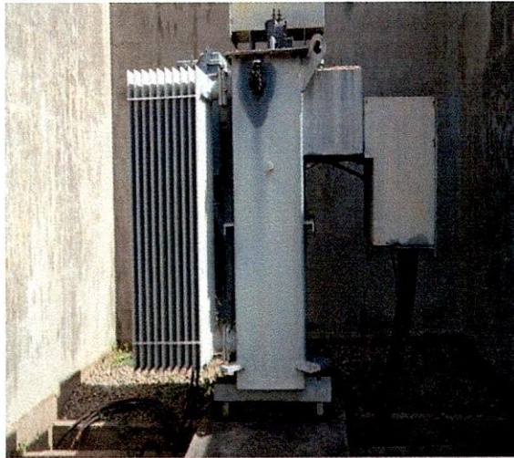
Moba LG-630KVA 33/0.415KV GEC Transformer, S.N.813681 Ekiti State Water Corporation I, Ero Dam, Ikun-Ekiti.
