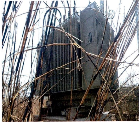
Moba LG-500KVA 33/0.415KV ABB Transformer, S.N. 1LPL407763 at Fountain Dairy, Ikun Ekiti.
