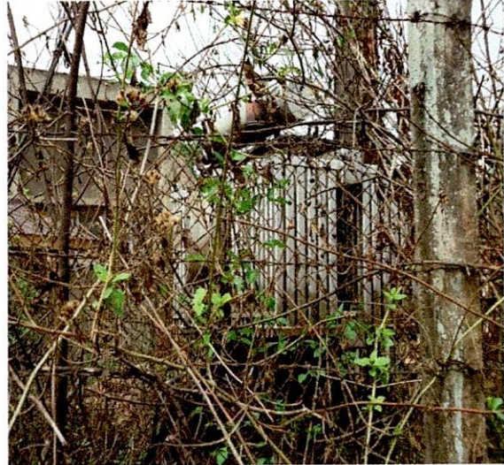
Irepodun LG-200KVA 33/0.415KV Elsewedy Transformer, S.N.1102000895 Ilawe Road Igede, Araromi Ekiti
