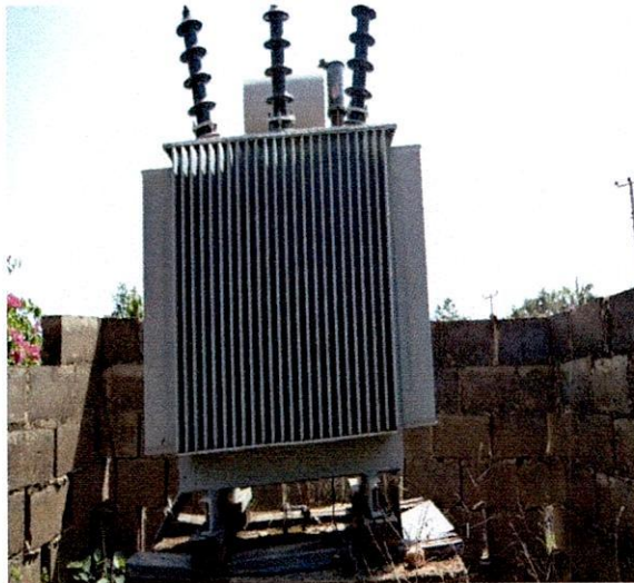
Moba LG-300KVA 33/0.415KV Enerco Transformer, S.N. 142244 In front of Justice Babalola, Omu Aran Road, Ekiti.
