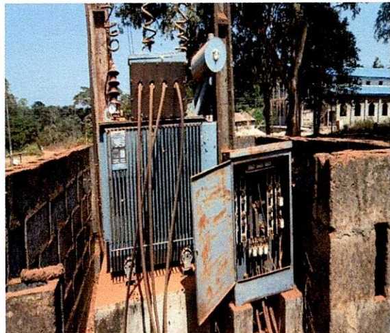
Moba LG-500KVA 33/0.415KV Mace Transformer, S.N. 49353 In front of Police Post, Osun Ekiti.
