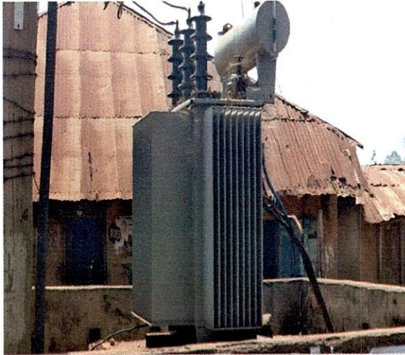
Moba LG-300KVA 33/0.415KV Pauwels Transformer, S.N.... Imuje Street, Otun-Ekiti.
