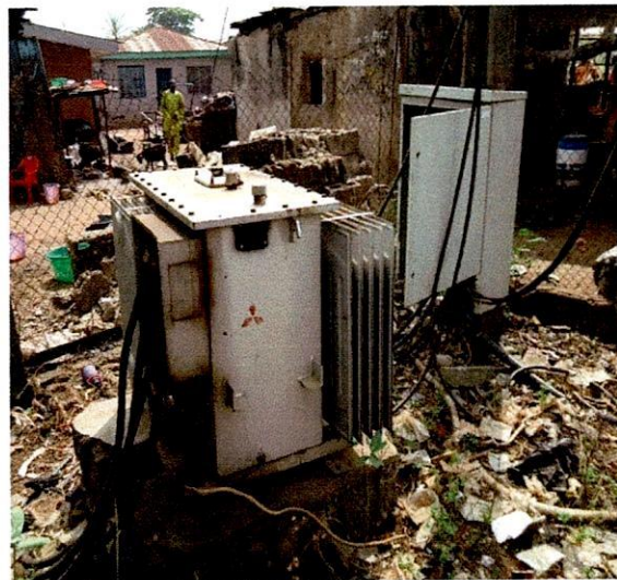
Irepodun LG-200KVA 33/0.415KV Mitsubishi Transformer, S.N.... Oke-Ilawe, Iyin Ekiti, Araromi Ekiti
