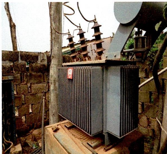
Irepodun LG-500KVA 33/0.415KV EFACEC Transformer, S.N.16610-09 at Unity Estate, Iloro Street, Iworoko, Araromi-Ekiti.
