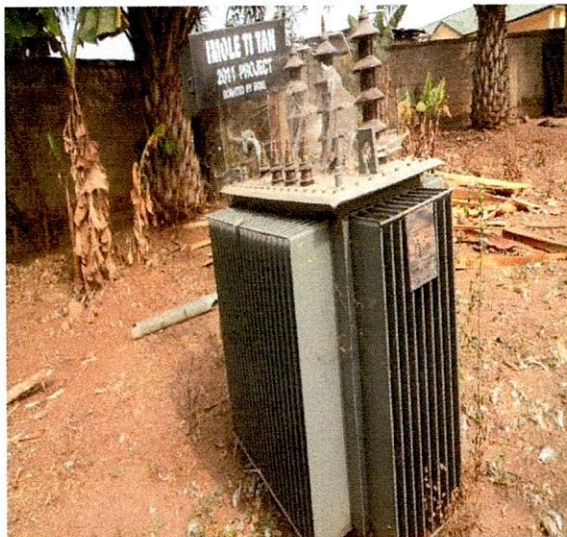
Oye LG- 300KVA 33/0.415KV Elsewedy Electric Transformer S.N. 1003000427 at Apeju Palace, Ilupeju.
