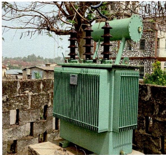
Irepodun LG-200KVA 33/0.415KV Koncar Transformer, S.N. 543855 in front of Anglican Church, Araromi Ekiti
