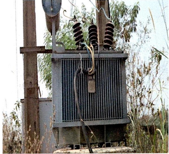
Ileje-Meje LG-300KVA 33/0.415KV Minel Transformer, S.N.107576 at Oke Okin Street, Iludun.
