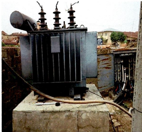
Irepodun LG-300KVA 33/0.415KV Elsewedy Transformer, S.N.0903000050 Odoleleyin Ilamoye Street, Araromi-Ekiti
