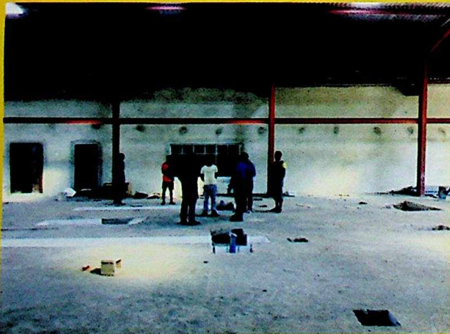
Ongoing works at Temple SYC computerized vehicle inspection project in Awka, to enhance road safety and vehicle worthiness in the State. The project is proposed to be commissioned during the third quarter of 2016
