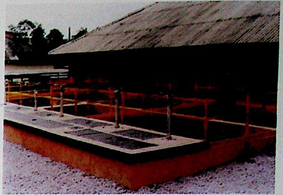
Eleyele Water Supply Scheme Filters
