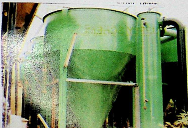
Asejire water supply scheme Sedimentation Tanks
