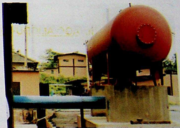
Eleyele Water Supply Scheme Surge Vessel
