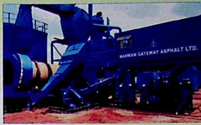
Gateway Asphalt Plant
