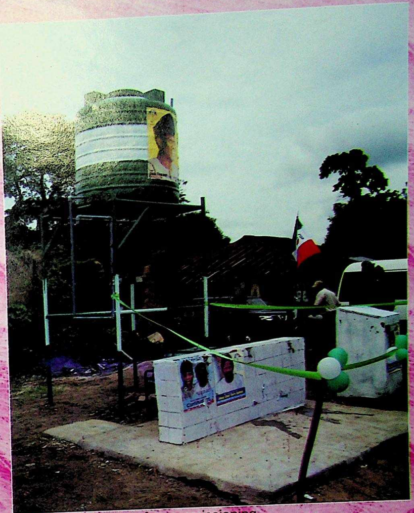
Water project ready for commissioning.
