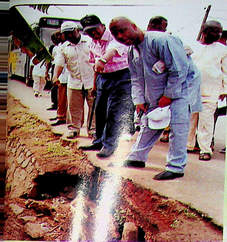
OGD and Special Adviser Works and Infrastructure, Engr. Kehinde Adeniji, inspecting a gully at a road construction site
