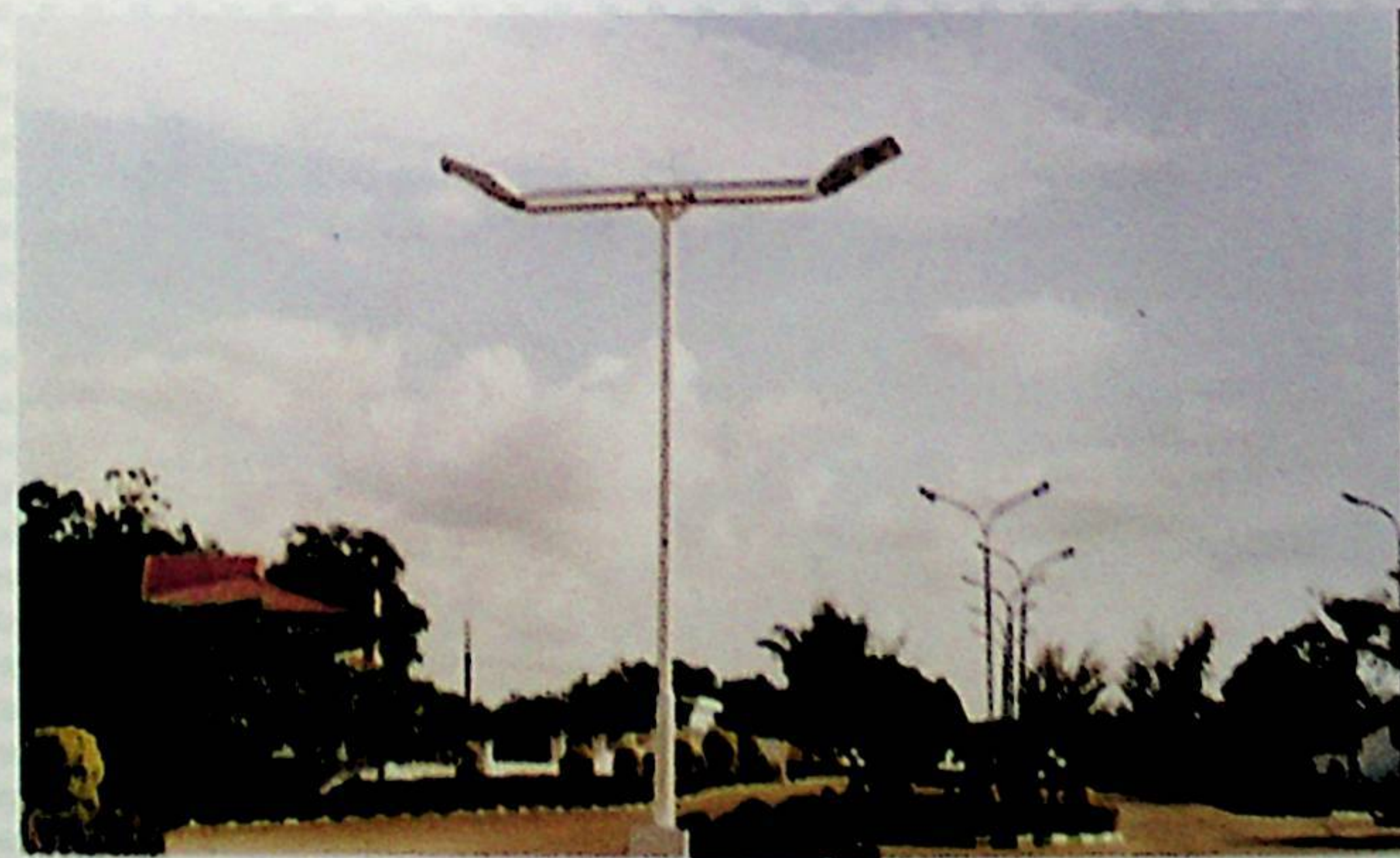
Solar energy for Street light
