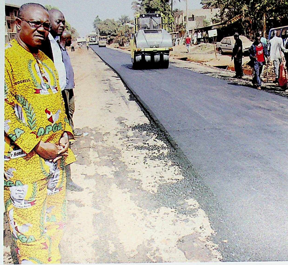
Governor Peter Obi inspecting the on-going construction of the Old Nkpor-Amawbia Road
