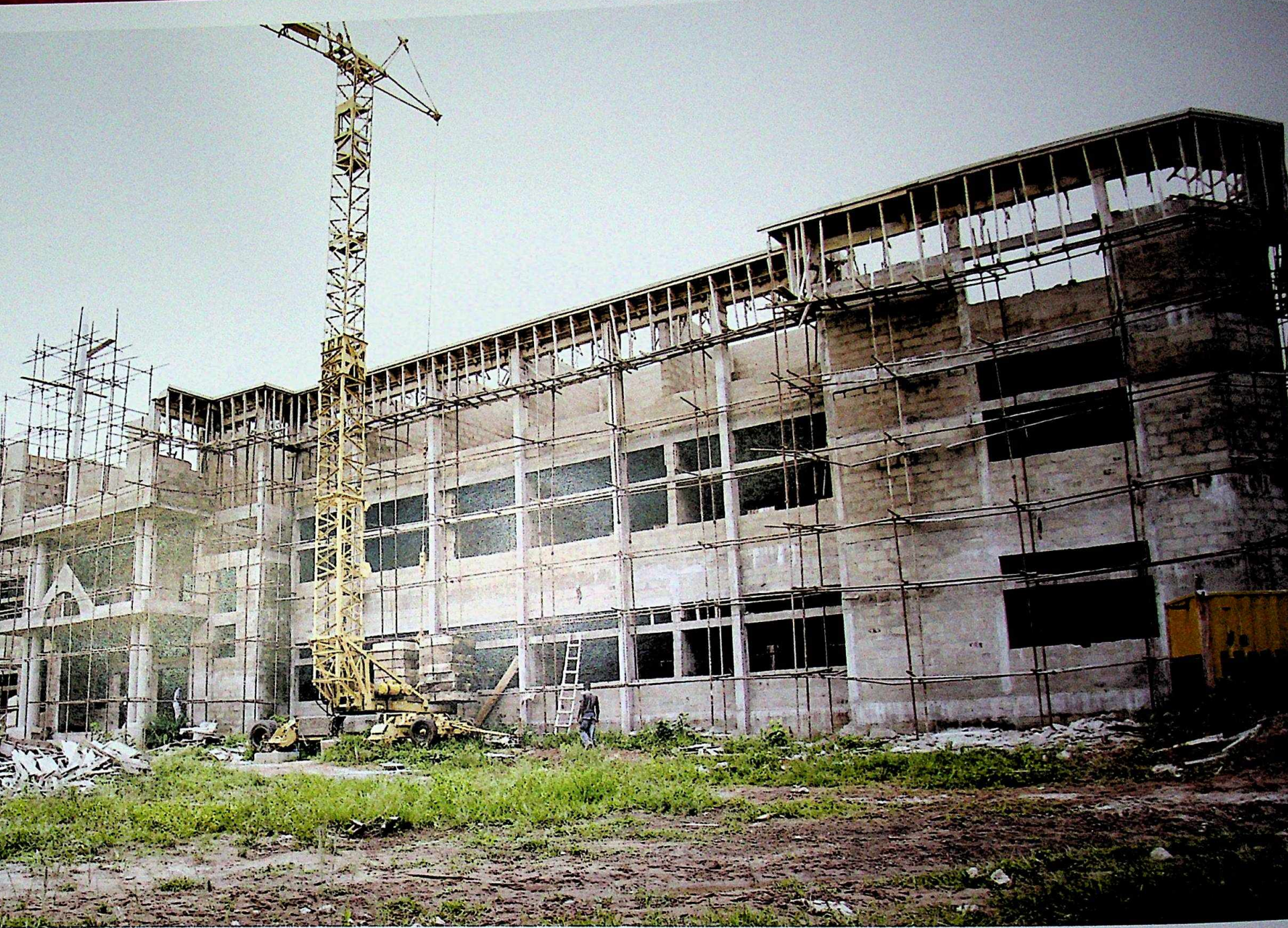
Faculty of Agriculture complex under construction at Igbariam Campus, Anambra State University
