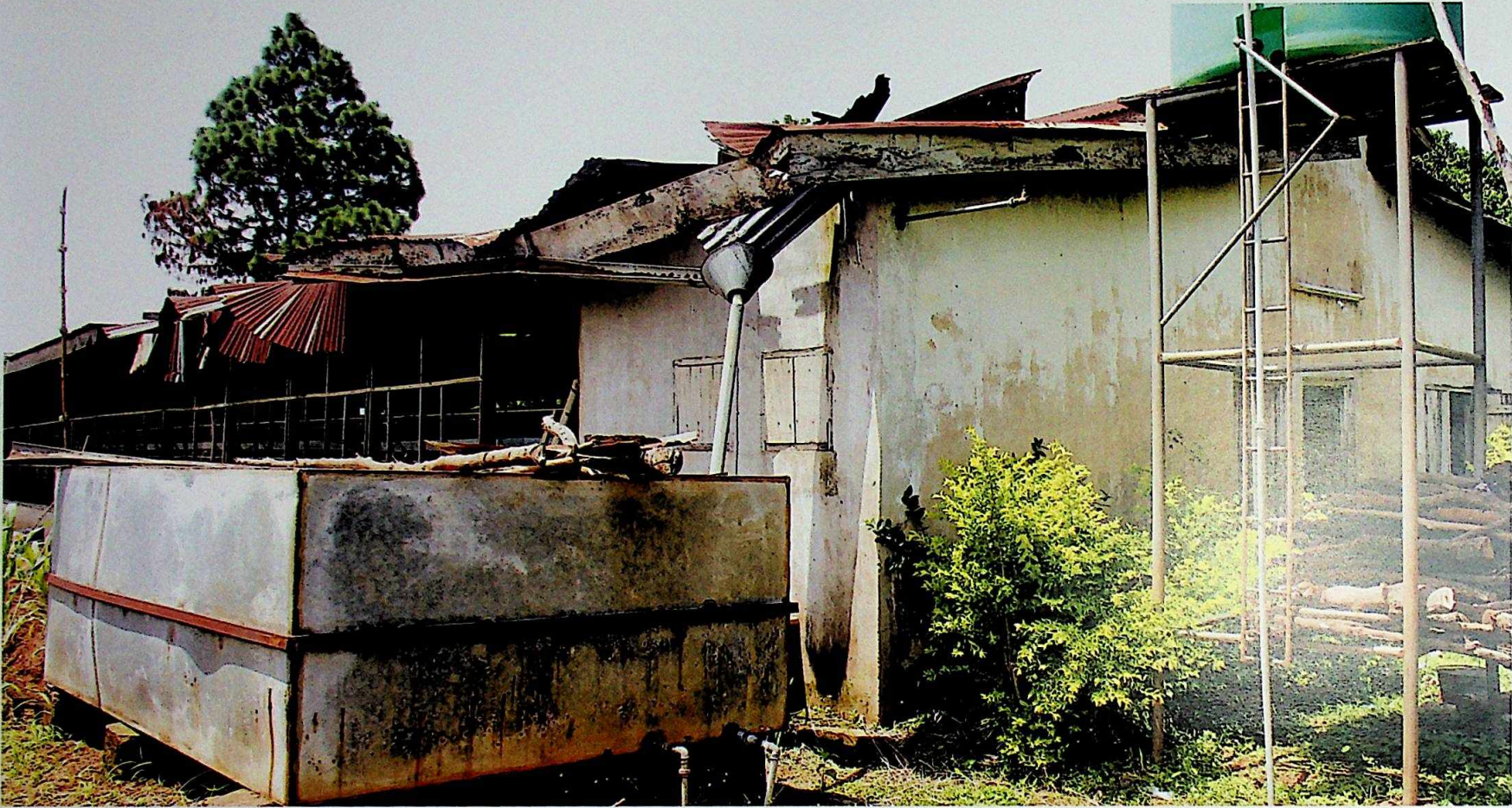
The old, dilapidated building depicting what the school used to be
