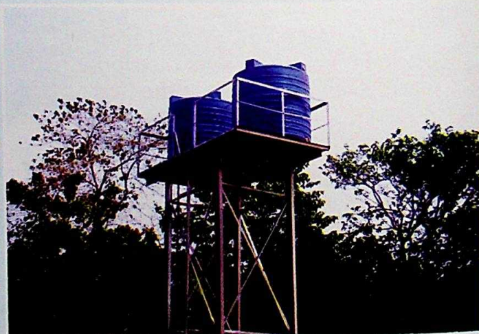
Motorized borehole provided
