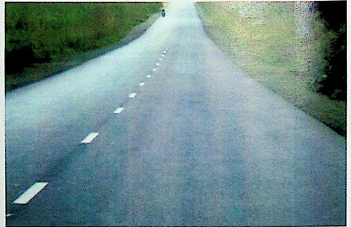
Completed 52km Section of Owelle Ezukala - Umunze - Umuchu - Amesi - Uga - Igboukwu Road
