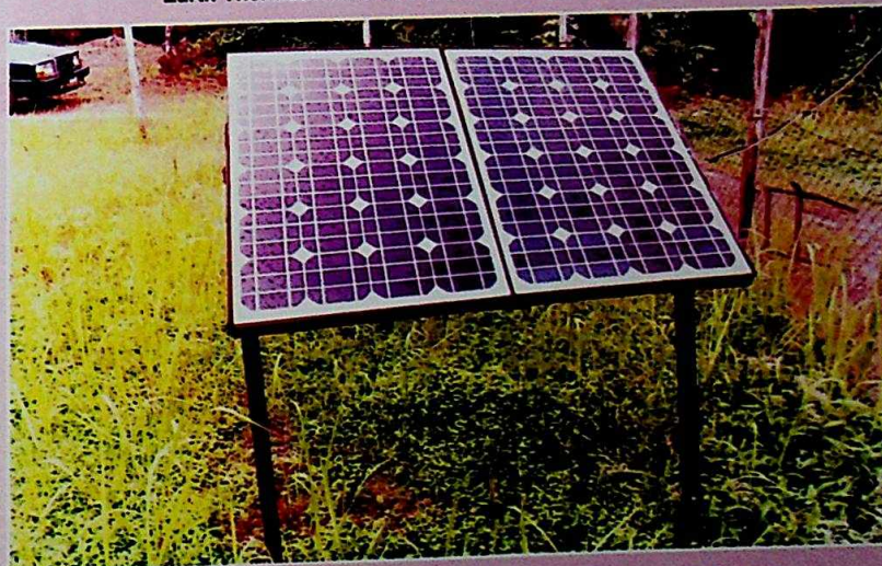
Solar Panel that attract energy which thereafter is converted to electrical for powering Meteorological Station
