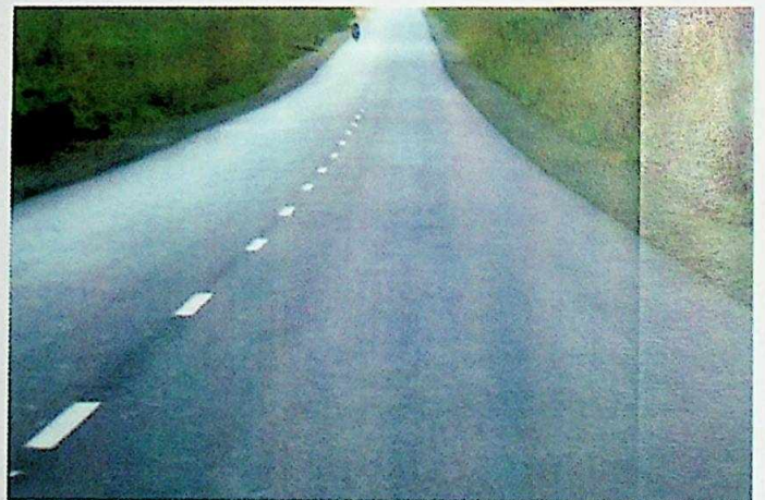
Completed 52km Section of Owelle Ezukala - Umunze - Umuchu - Amesi - Uga - Igboekwu Road
