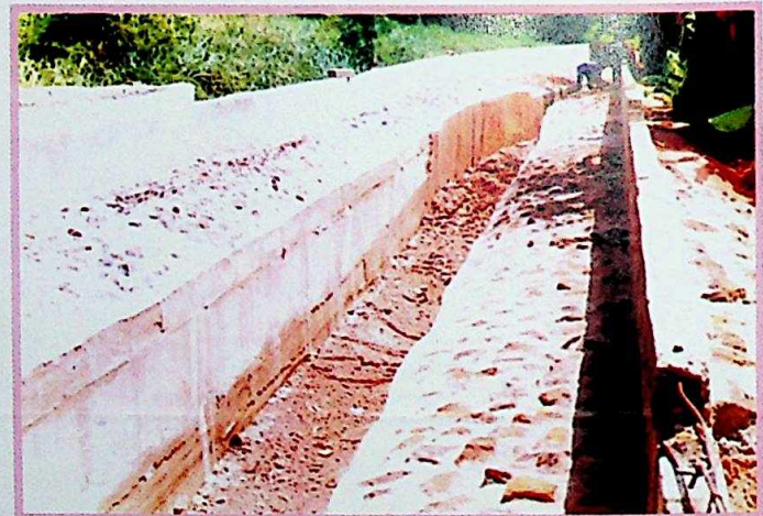
Technology incubation centre Nnewi erosion site after intervention measure.
