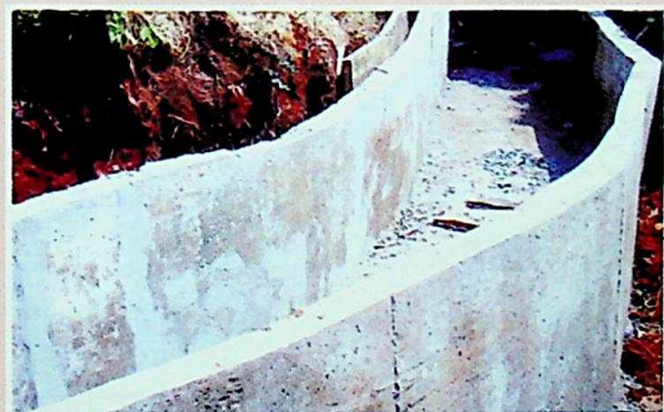
Completed reinforced concrete drainage channel from the source of the cause of the gully.
