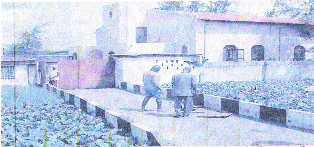
The Dispensational Gospel Church building with culvert built across the McGregor Canal and impeding flow of channel
