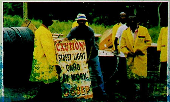
One of the streetlight gangs created by OGSEP to accelerate pace of work across the state.
