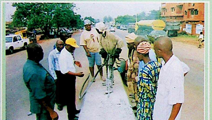
Engr. Olufolaranmi Onayemi leads other top funtionaries of OGSEP on inspection visit to project site on Awolesi Road, Sagamu.
