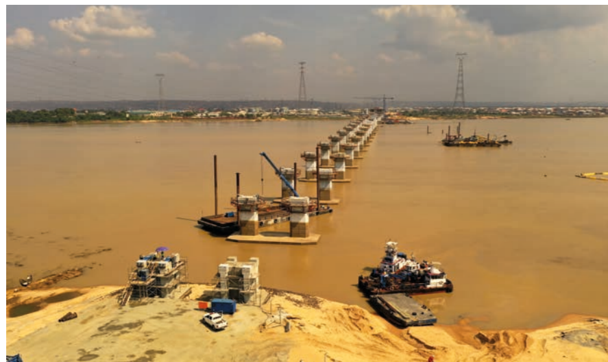
Completed Piers of the 2nd Niger Bridge - View from the Western Approach.
