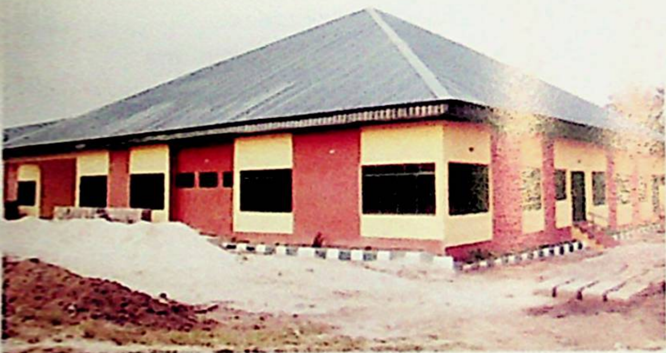
Model Primary School at Kur, under construction communal clash or youth restiveness which usually results in the loss of lives and properties in the area".
