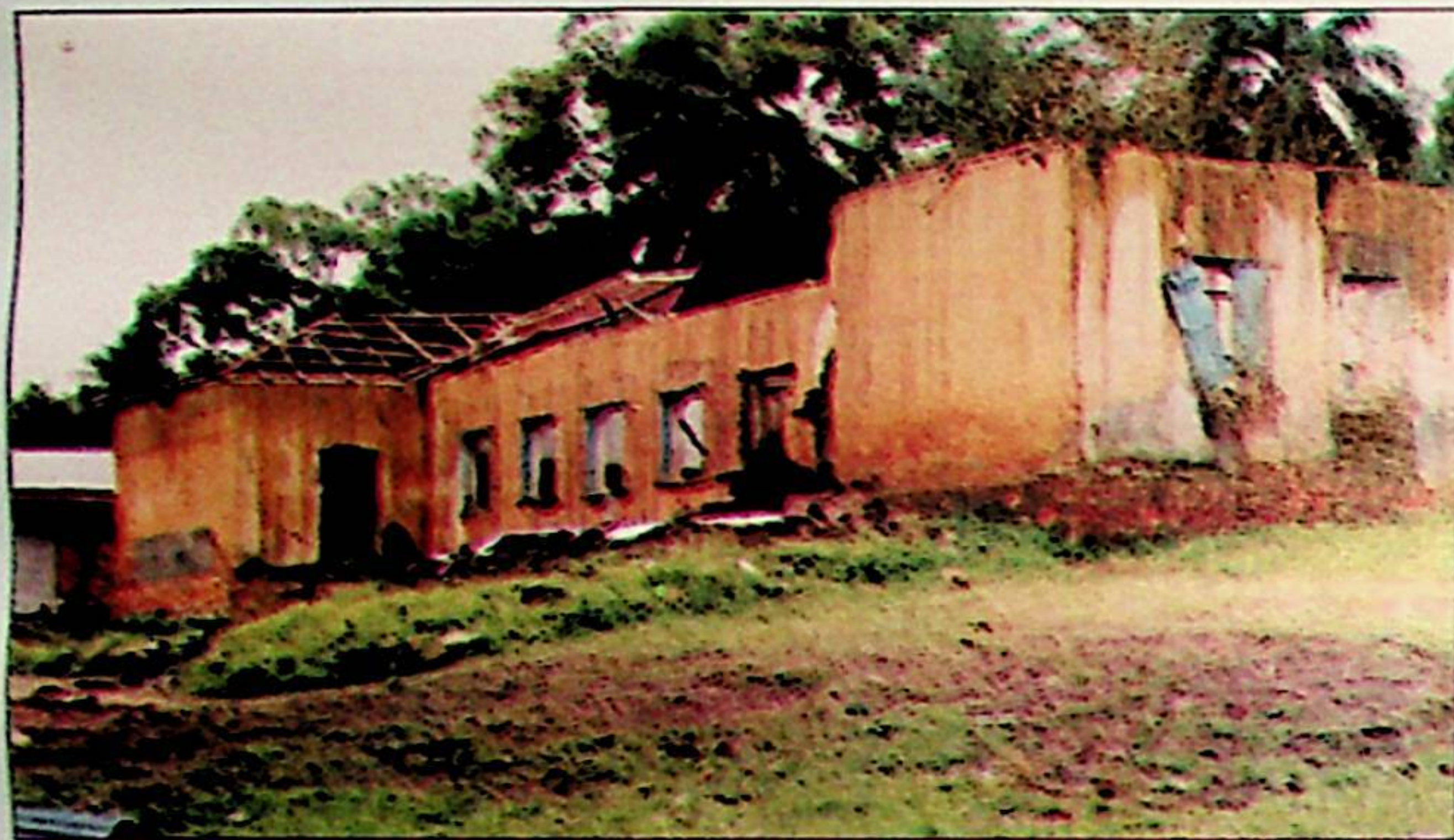
Dilapidated school used during the Last administration
