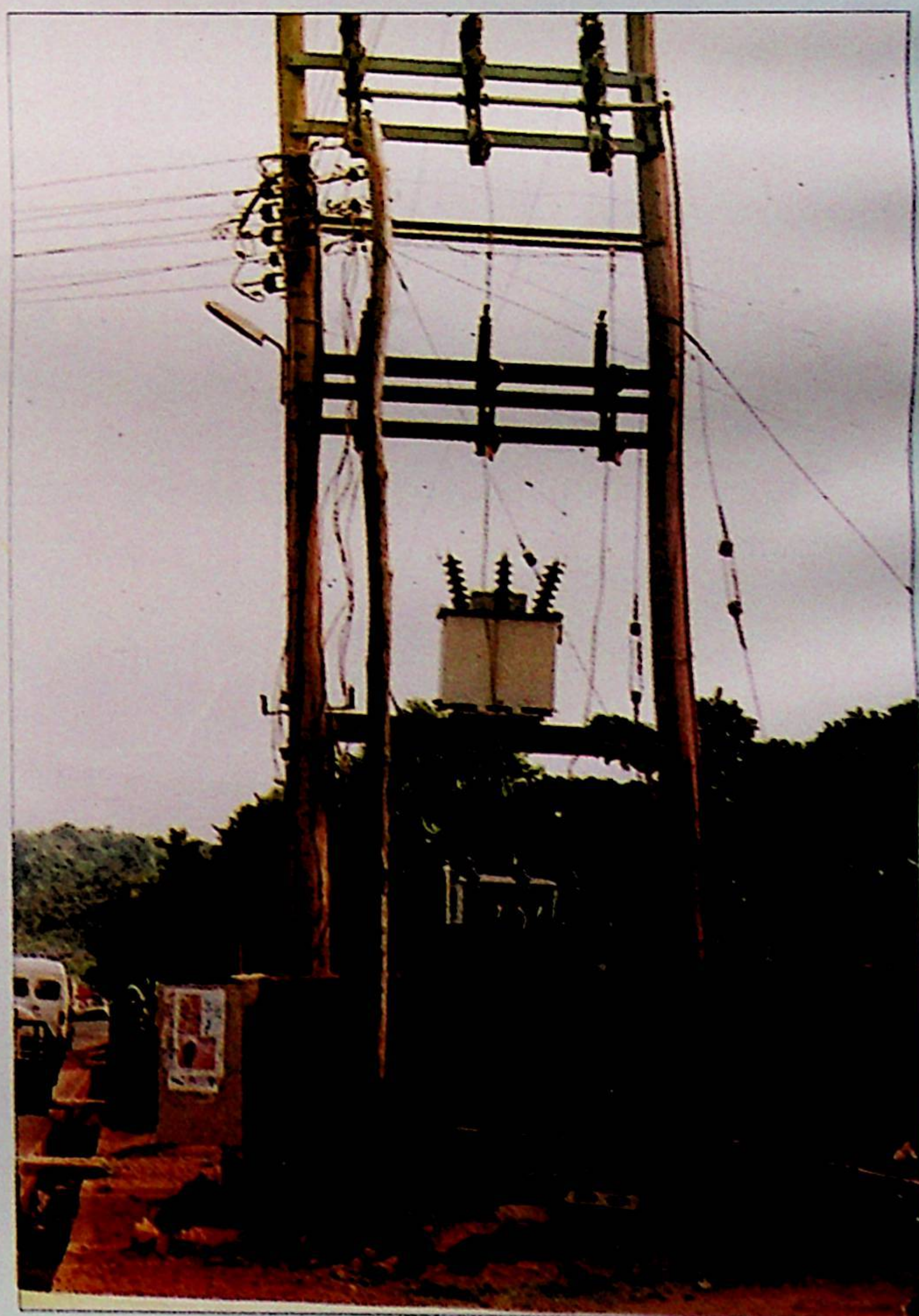
Transformer point at Ikuehi-Ihima Okehi LGA
