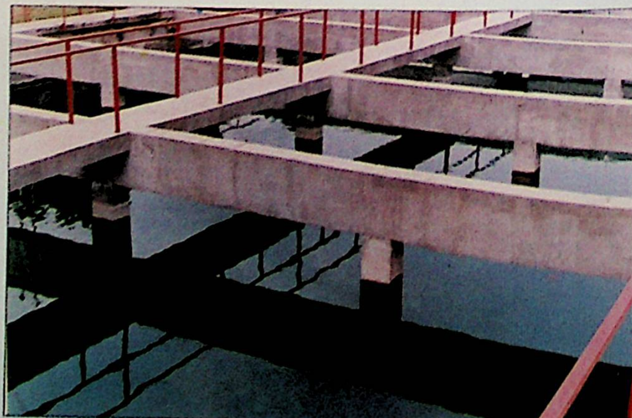
Idah Water Works Sedimentation Tank
