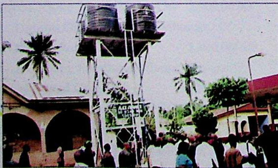
Bore Hole Powered by Solar Energy
