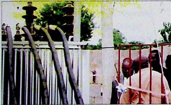
Electricity at Ezi-Orsu, Oguta LGA.
