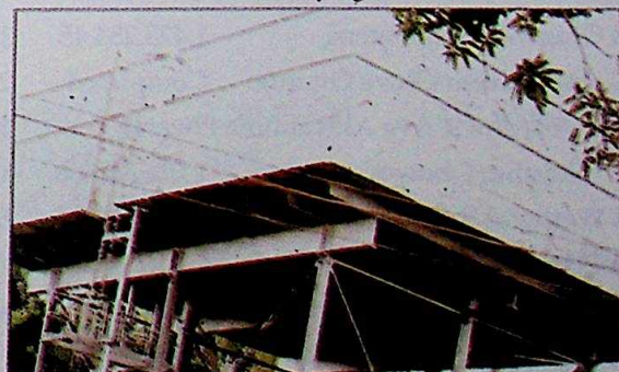
Overhead Tank at Atta Njaba Water Scheme
