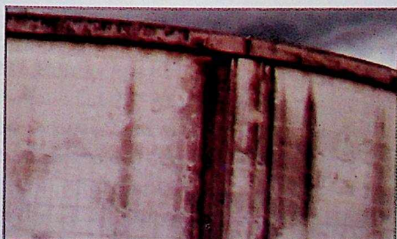
Tank at Egbeada Water Scheme
