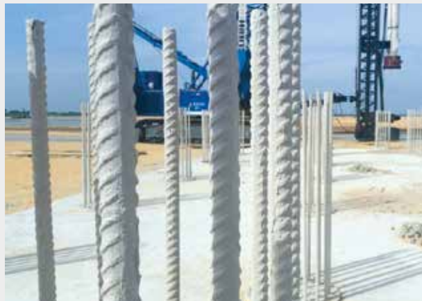
EW III, Ongoing construction at the site of the Second Niger Bridge.
