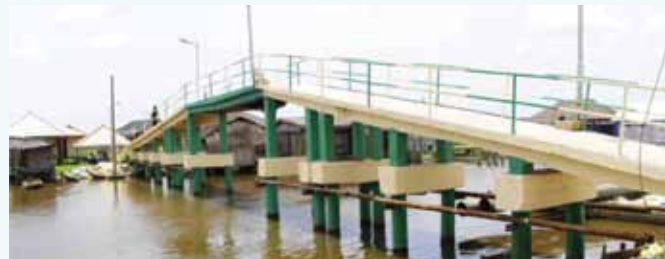
Concrete Pedestrian Bridge with 800meters Concrete walkway, Tsekelewu and Pinakiri Zion, Warri North L.G.A.
